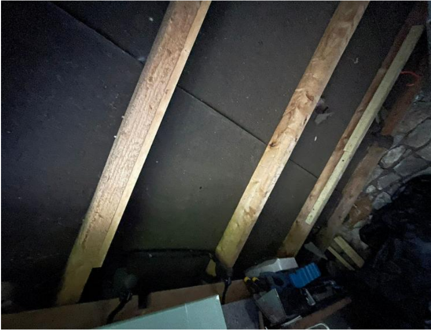
Photograph 3. Internal view of the Bitumen-type liner below the roof tiles with tears and holes.
