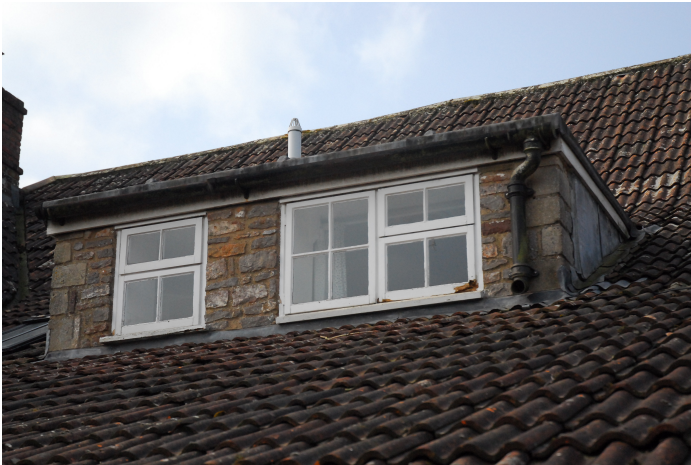
Fig.5 Dormer windows with bird damage
