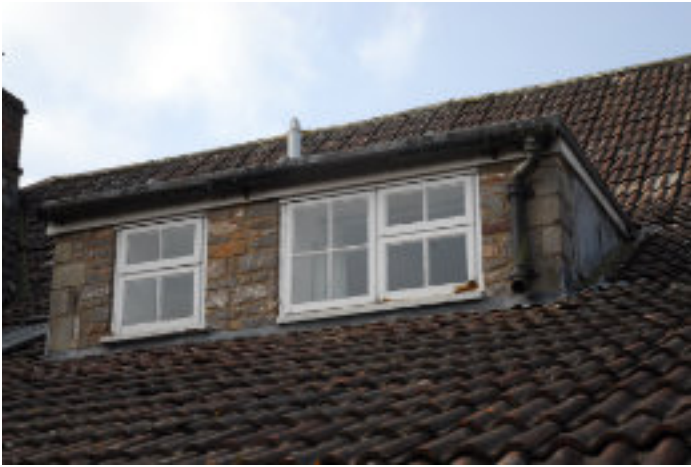
Fig.5 Dormer windows with bird damage
