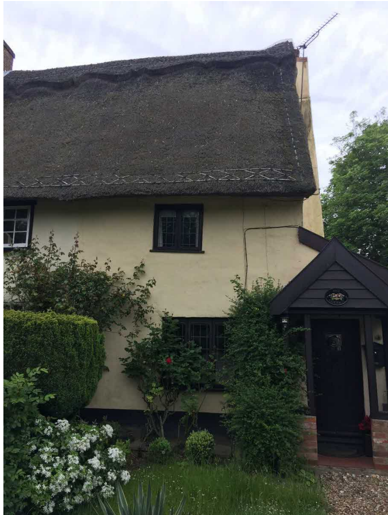
Fig. 3: Front elevation showing windows to ground and upper floors, both c.1980 casements, and entrance porch
