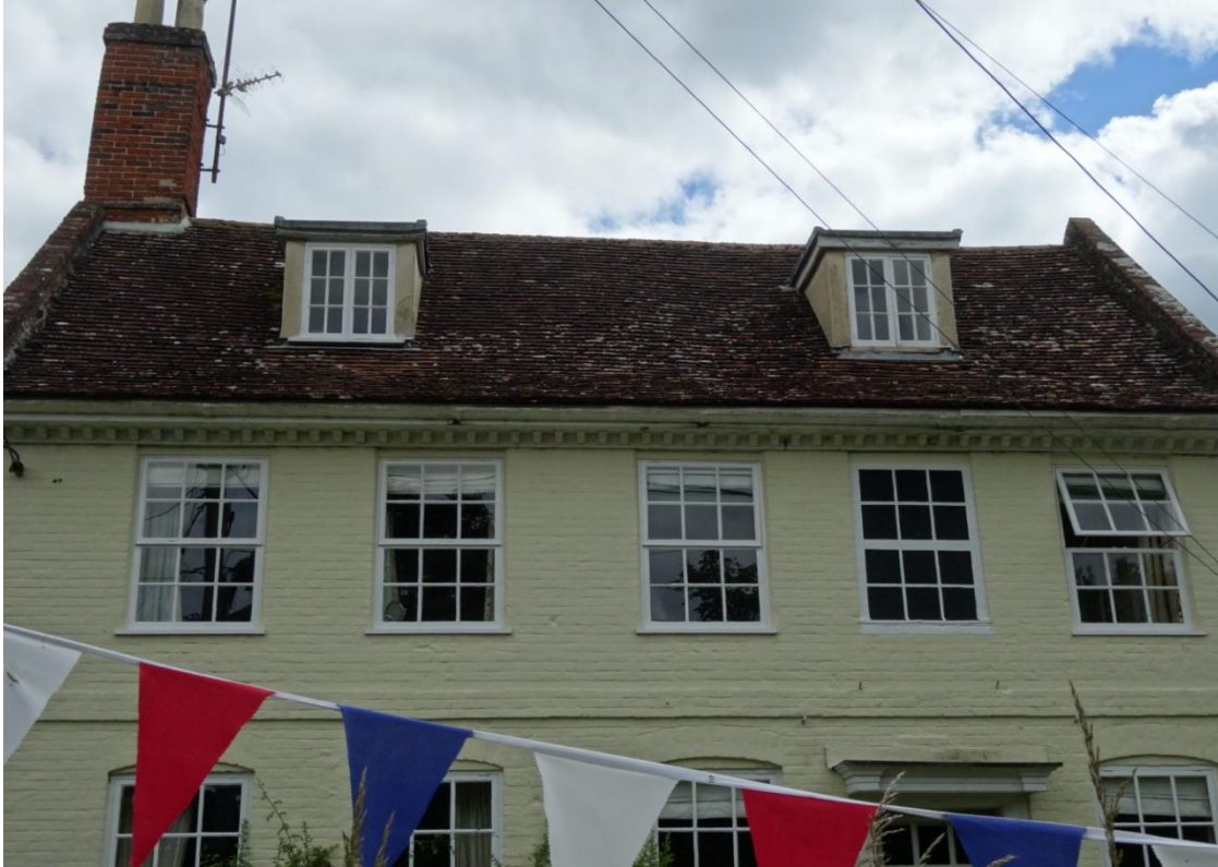
Front view of house with dormer windows at the top of the house which need replacing.
