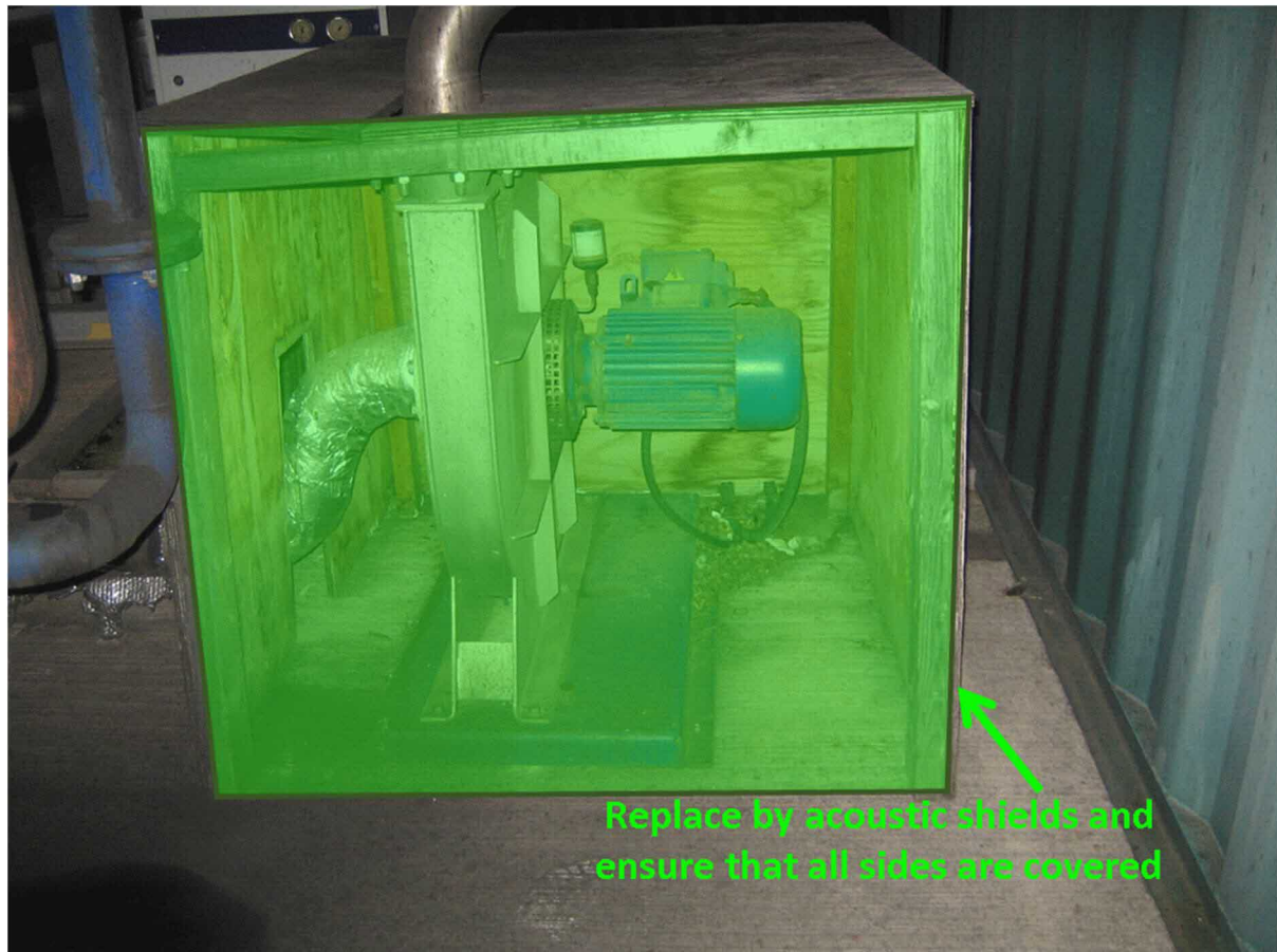
Figure 18 Improved enclosure around gas booster fan
