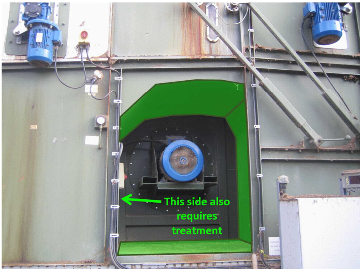
Figure 11 Shields location in motor recess (green)
