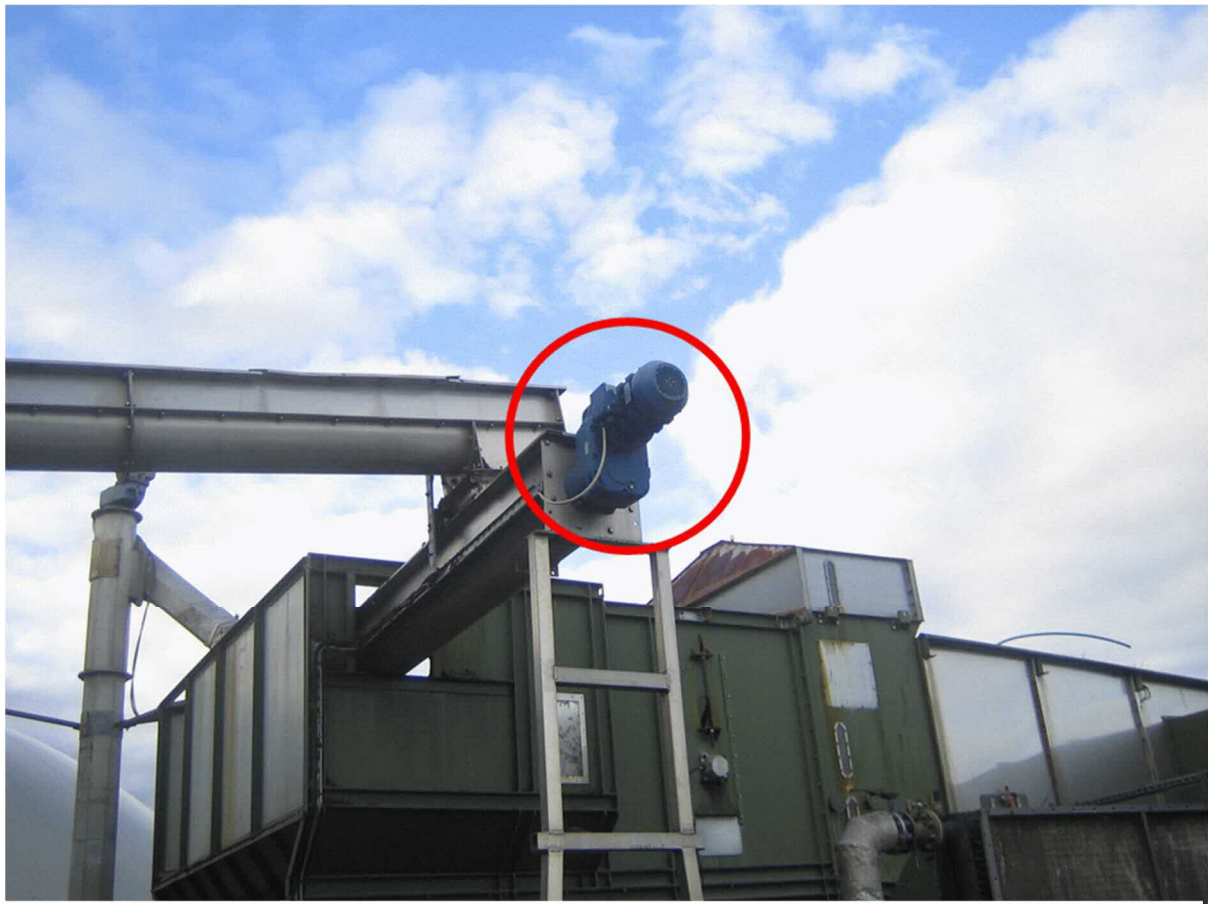
Figure 10 Dryer fan infeed conveyor motor
