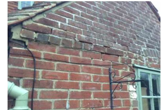
15. Unstable structure which is could affect the Heritage asset.
