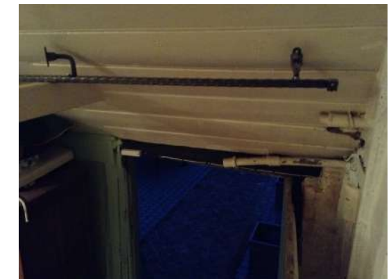
16. The roof timbers are rotten and losing support.
