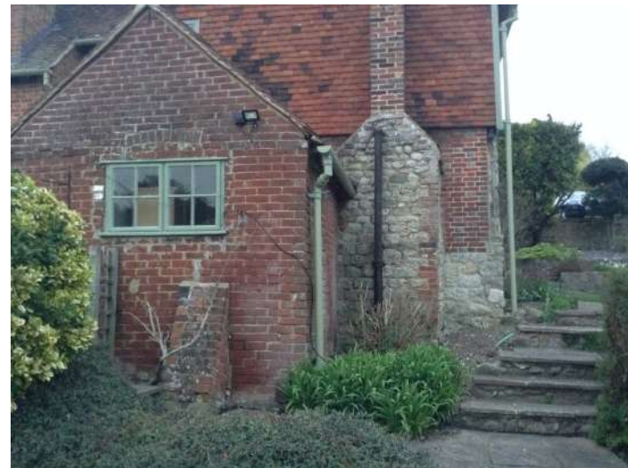
8. Existing ground floor brickwork is bulging and has been repaired in cement and buttressed for support.
