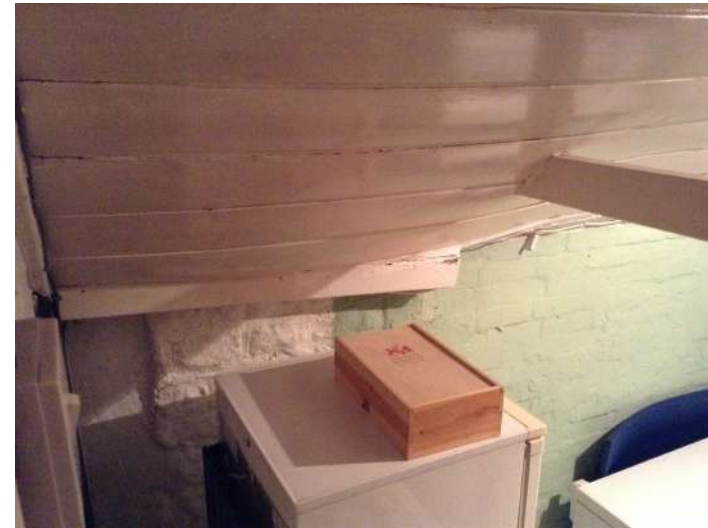
6. Existing north-west, ground floor side structure is in a state of decay and collapse.
