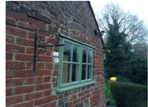
14. Bulging brickwork with cement repair
