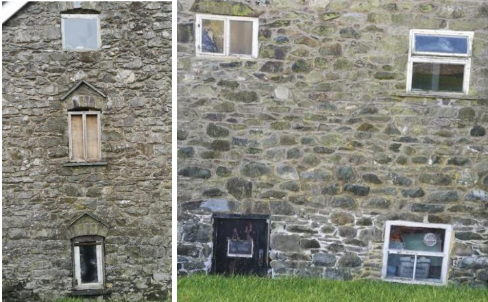
Existing condition of original casement windows [ref D] to the north and west elevations
