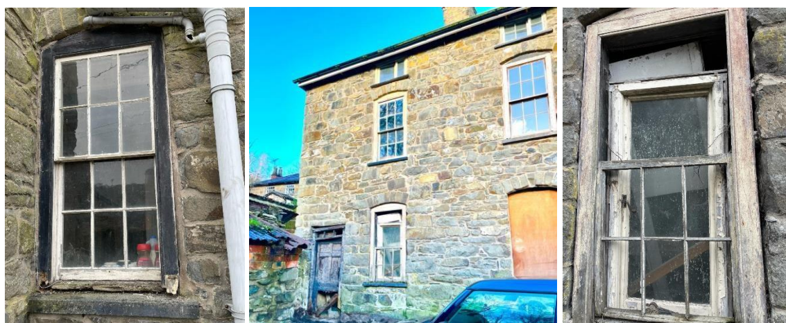
Existing condition of original sash and casement windows [refs A, B and C] – principally to south and east elevations. [Note: existing grey PVC SVP and pipework to be replaced with black UPVC].
