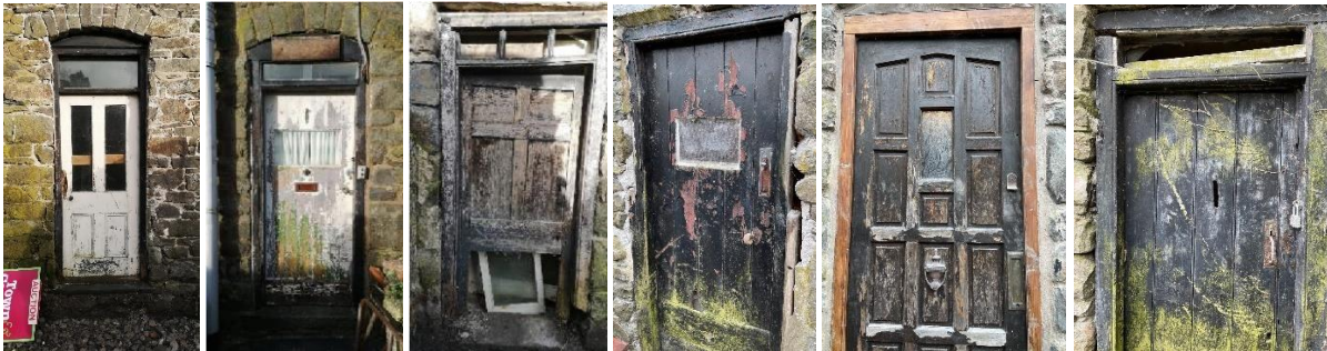
Variety and condition of existing non-original external doors [3no to front, 3no to rear]
