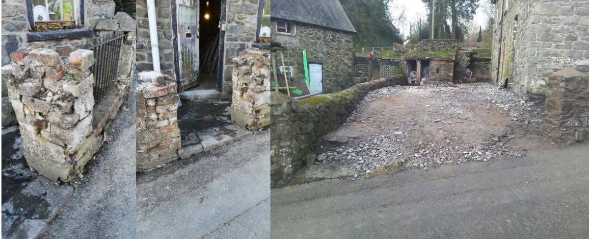
Condition of existing piers to wall and the removed wall proposed driveway [incomplete]
