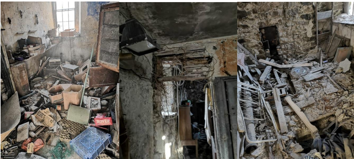
Dilapidated Interior to Cottage no. 3
