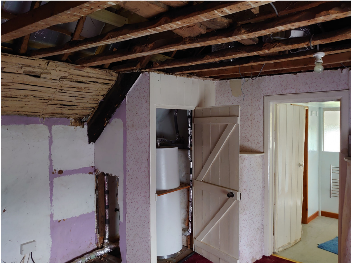
Fig 8 showing cylinder cupboard to be removed and collapsed ceiling.
