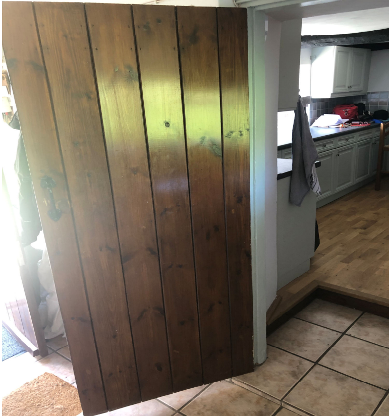
Fig 2 20 th C Door between rooms 1 and 2 showing 2 unequal steps within wall thickness.
