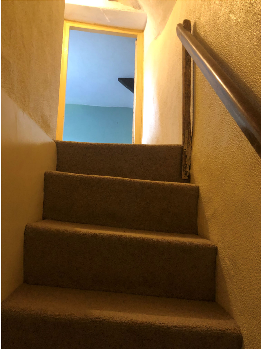
Fig 11 showing stairs with dangerous unequal treads and risers. Line of later partition on left visible at upper floor level.
