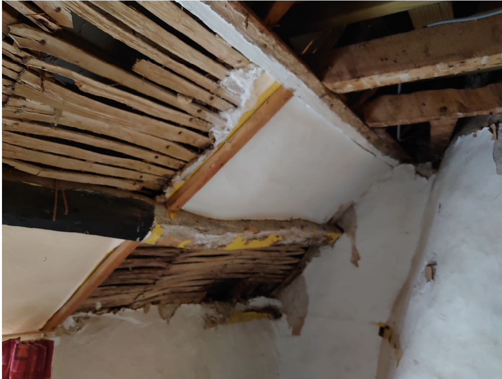
Fig 9 showing collapsed ceiling beside chimney gathering in room 9.
