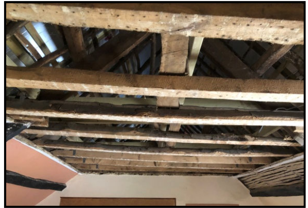
Collapsed ceiling: image 3.0
