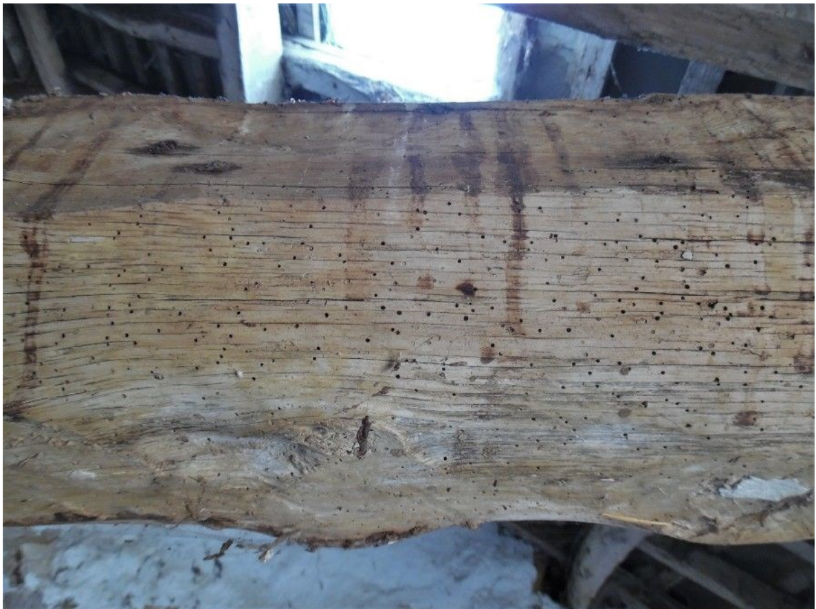
Plate 8: Insect boring attack of timber roof truss.
