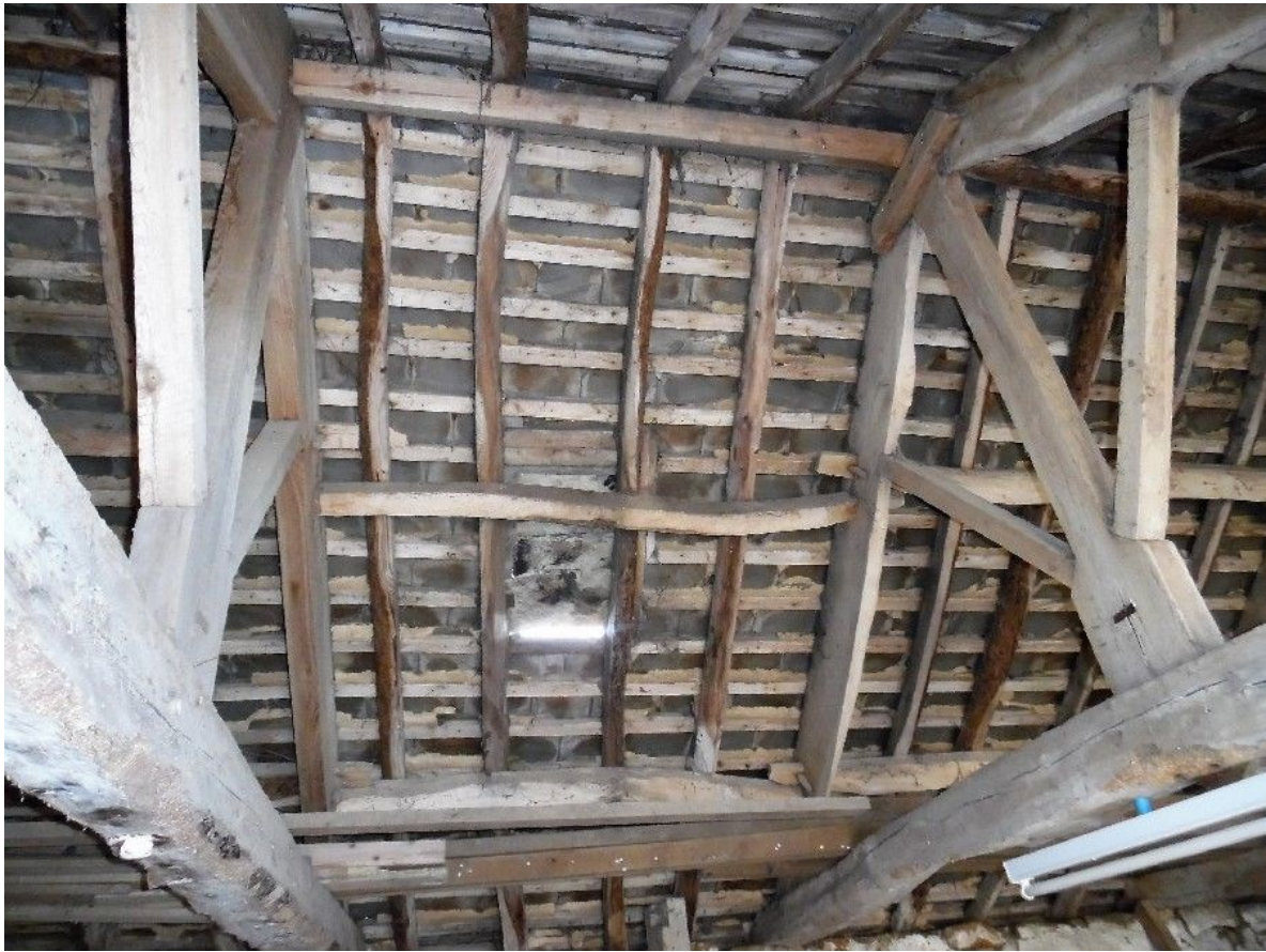
Plate 5: View of the barn roof. Note bent purlins, possibly tree branches or small trunks.
