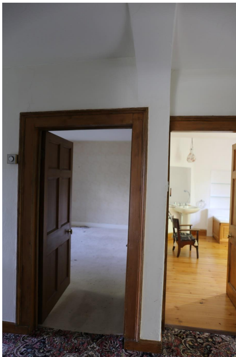
Plate 20: First floor bedroom doorway at first floor level, cutting into the archway above, possibly redesigned from the original
