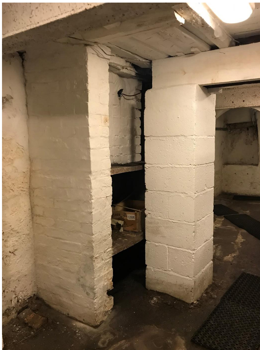
Plate 28: Substantial stone flag shelving in the basement, courtesy of Studio SDA Architecture.
