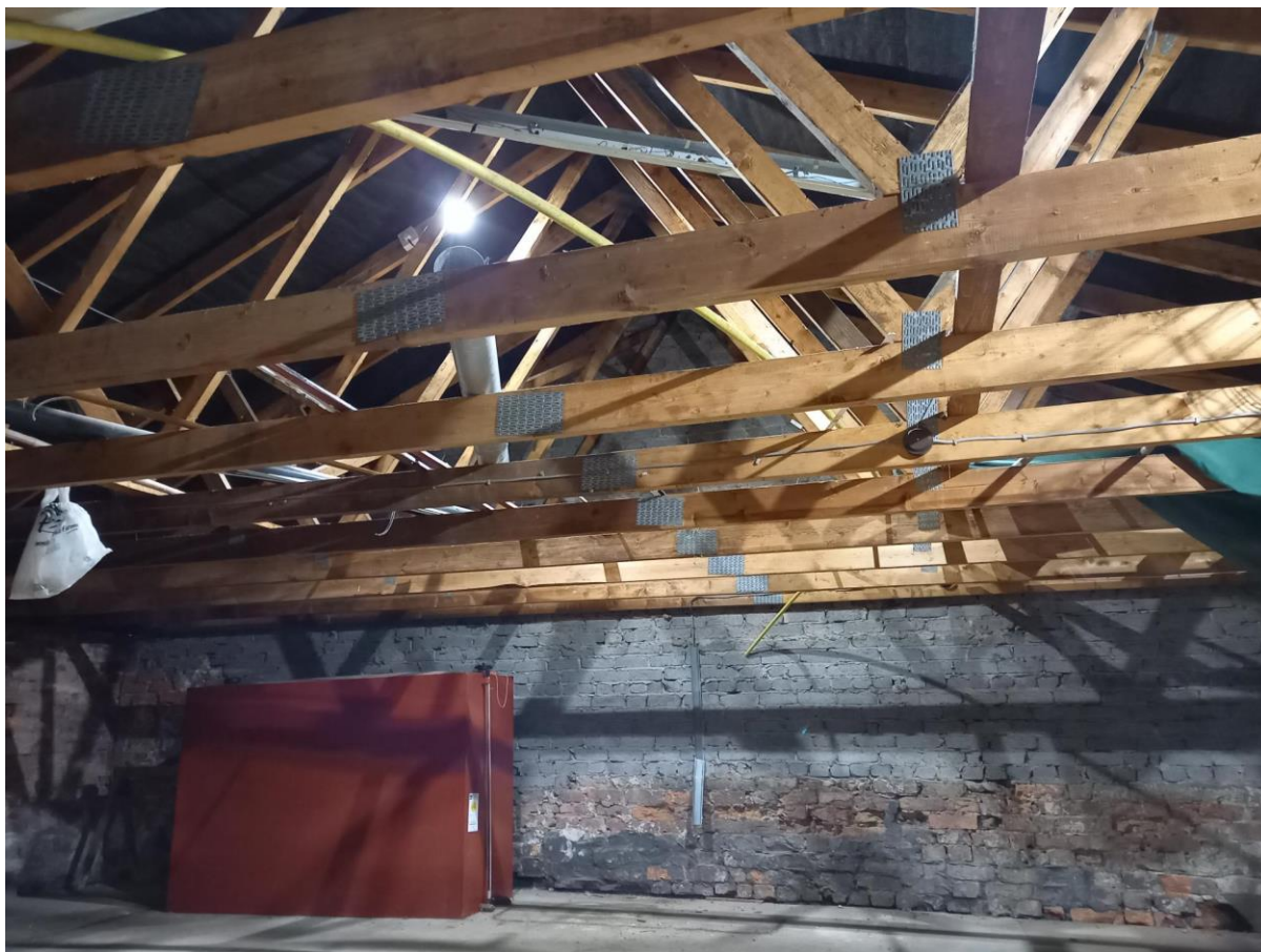
Plate 33: The roof frame is clearly very recent, courtesy of Studio SDA Architecture
