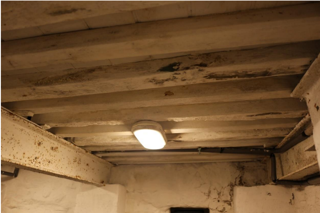
Plate 25: Ground floor joists above the basement, carried over modern piers and sections of reinforced steel joist
