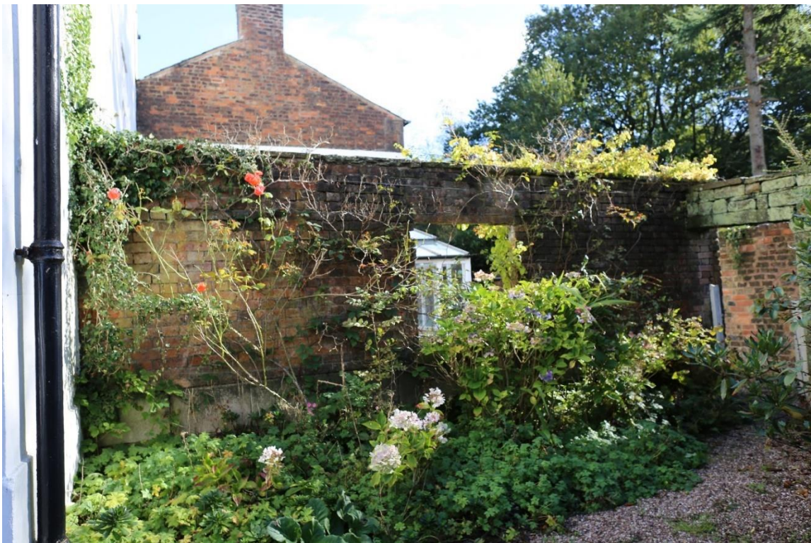
Plate 40: A section of the eastern wing which survives only as a standing wall with window opening
