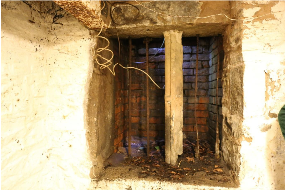
Plate 29: Window or hatch entrance with central mullion on the west side of the basement next to a drain sump.
