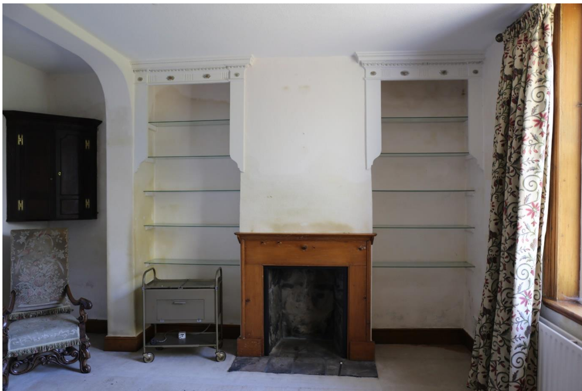
Plate 13: Chimney breast, fireplace, cupboard and window frame in ground floor dining room
