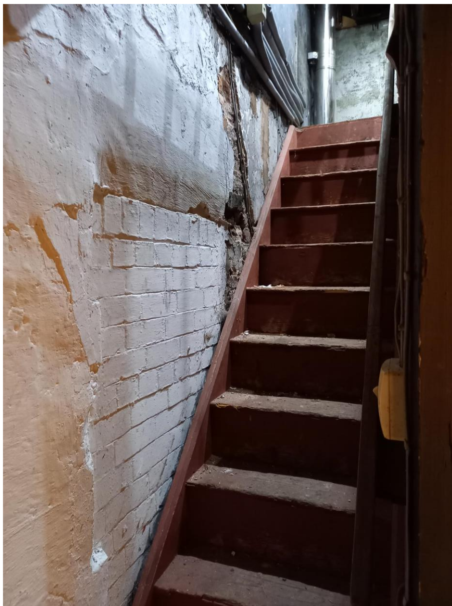
Plate 34: Steps up to the first floor reveal the location of a blocked doorway, courtesy of Studio SDA Architecture
