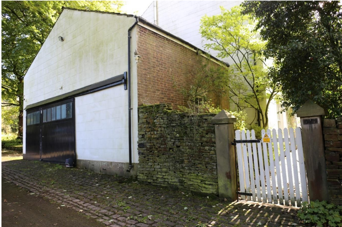
Plate 31: Western wing external elevations, facing east. Note unrendered brick, section of stone wall and sliding garage door.
