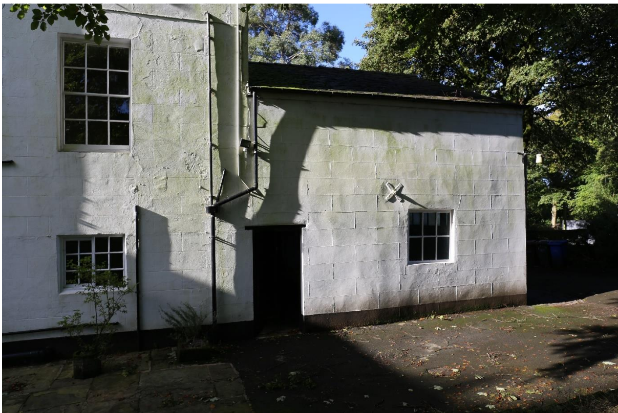
Plate 30: Western wing, now garage and utility room. Note stone block effect render over brick and tie bolt.
