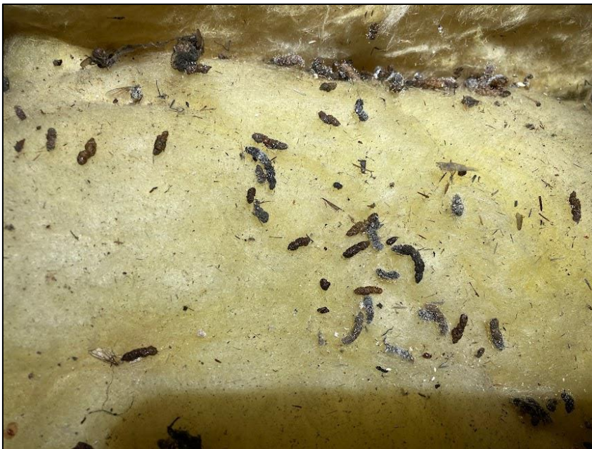
Photograph 21 showing bat droppings found in the roof void space
