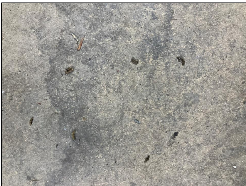
Photograph 25 showing the scattered bat droppings found in the garage
