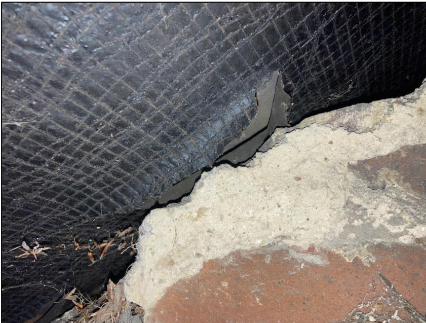
Photograph 19 showing one of the rips in the roofing felt
