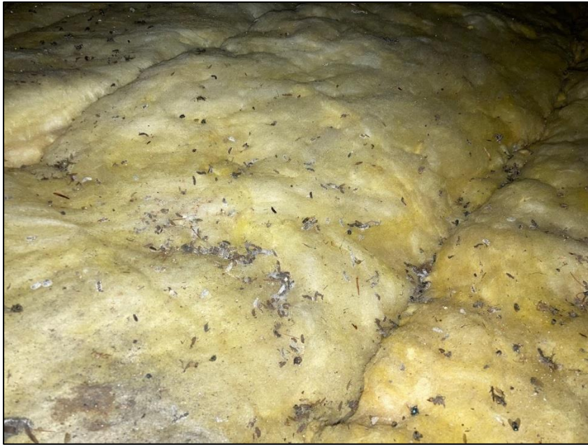
Photograph 20 showing bat droppings found in the roof void space
