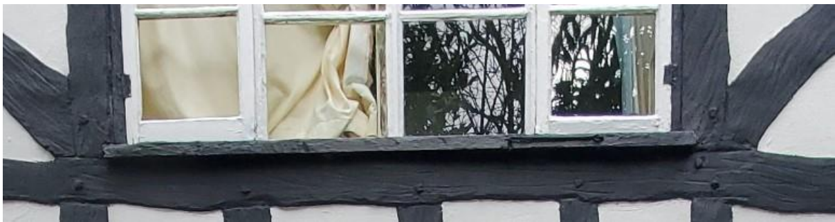
Picture showing damage to window 4 – Second floor side wall
