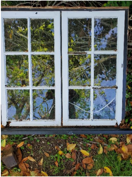
Picture showing design of and damage to current windows 1,2 and 3
