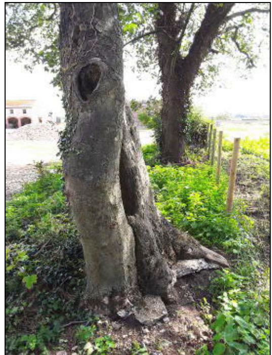
Large sections of concrete are embedded in the base of T5; basal decay is evident, particularly on the north and west sides of the tree
