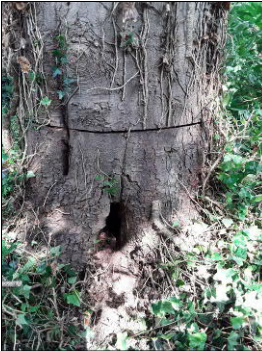
T2, a category "C" tree has a decay cavity in the base of the tree and has been ring-barked in an attempt to manage the ivy coverage
