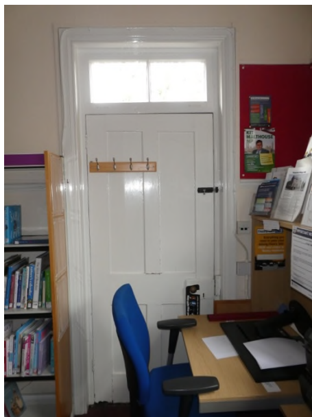
Figure 33: Part-glazed panelled door with overlight on the LHS of the west elevation of G13
