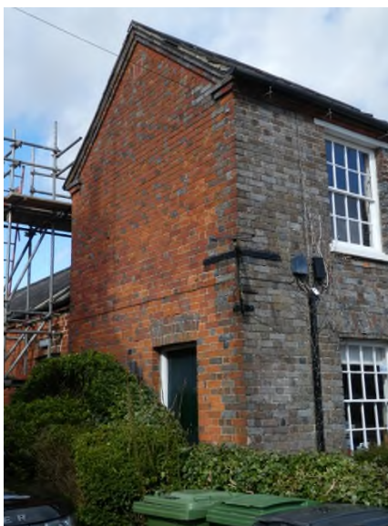
Figure 2: Oblique view of the west gable end elevation of the Phase 3 extension
