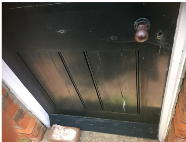
Figure 17: Detail showing the crisp finish of the panels of the door on the west elevation of Phase 3
