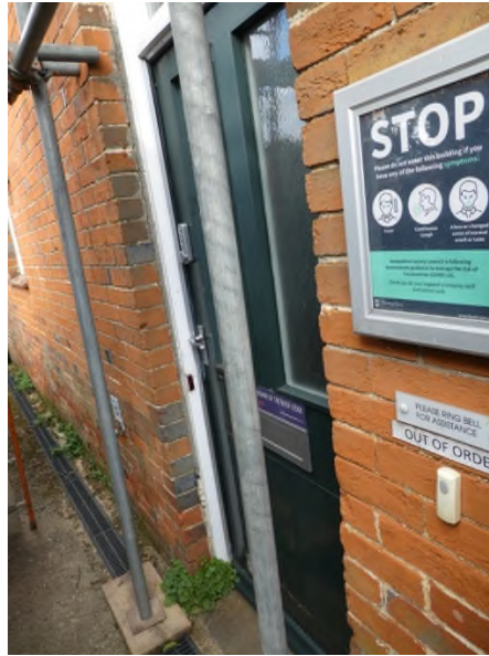
Figure 18: Existing door on the right hand side of the west elevation of Phase 4
