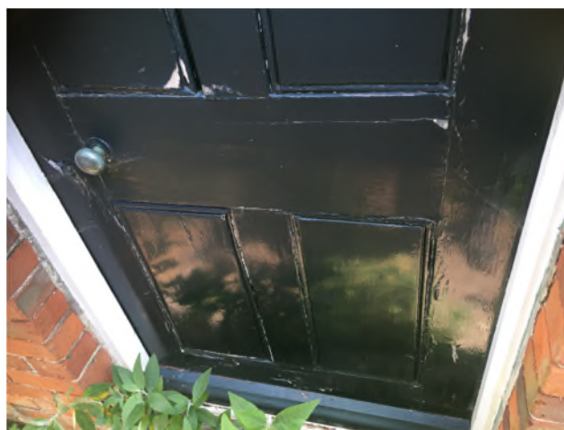
Figure 21: Detail of the panels of the original door on the west elevation of Phase 4
