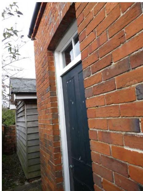
Figure 20: Original door on the left hand side of the west elevation of Phase 4
