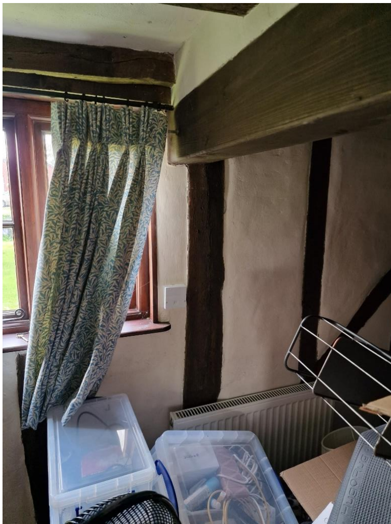
Northerly wall. Modern beam housed in wall where chimney stack once was.
