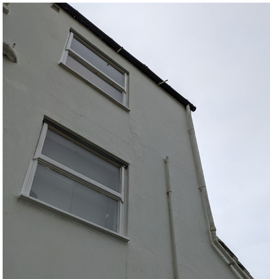
Existing photograph of poor quality glazing that is proposed to be replaced to match the original
