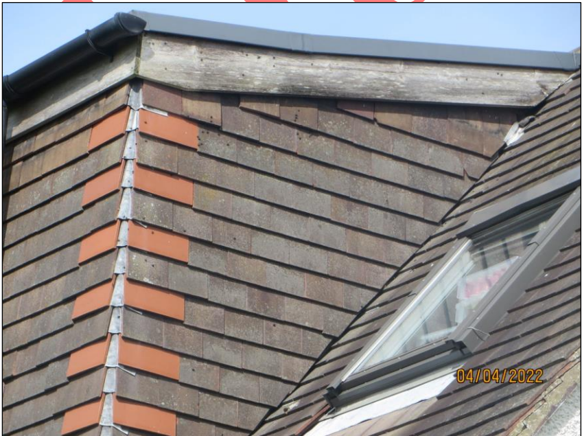
Figure 10. Gaps present around dormer window.
