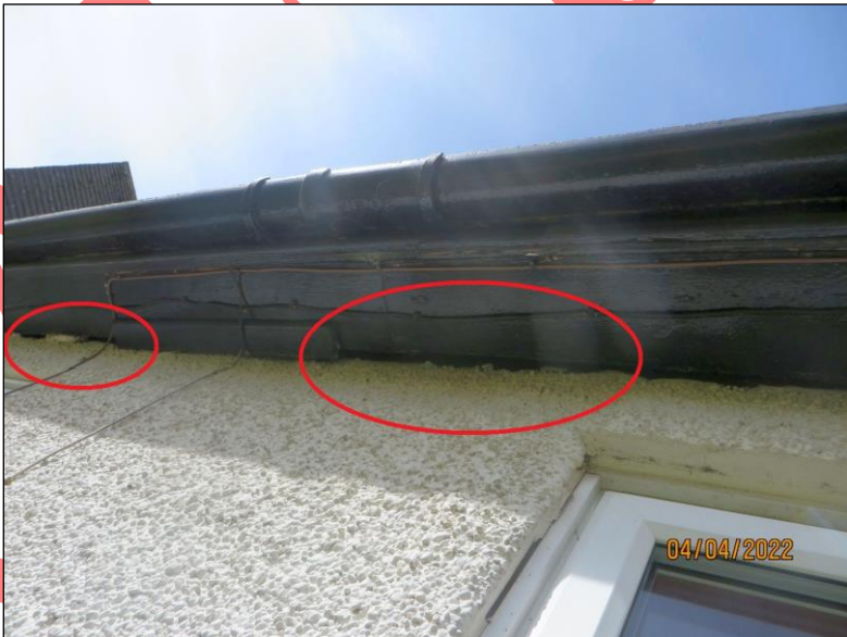
Figure 9. Gaps present into soffit boxes.
