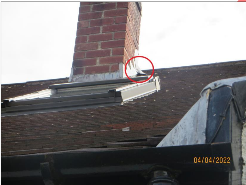
Figure 12. Raised roof flashing.
