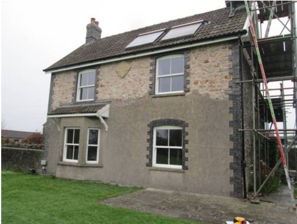
Picture ref 02 – Side South Elevation of House as Existing – render being replaced (November 2020)
