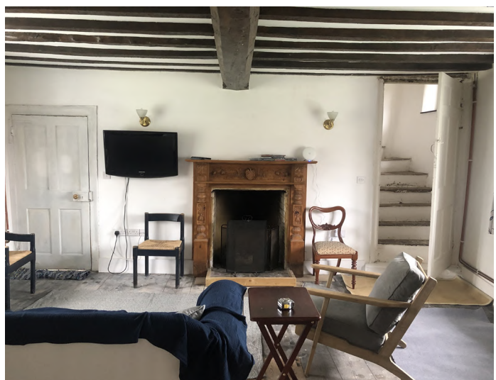
Proportions of the fireplace opening, over-elaborate and crudely carved fire surround and its off-centre position clearly indicate its later date. Winder stairs to the right lead to the first floor and attic level.
