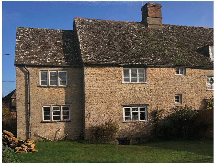
Rear of Rose Cottage taken in November 2014 prior to the partial implementation of the 2010 scheme which included a single storey extension and the insertion of two dormers, one in the older section of the building and the other on the later subservient range. All the windows have subsequently been replaced.
