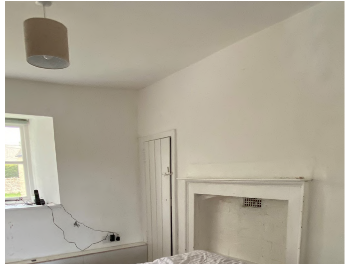
A small section of stone moulding is discernible just below the later fire surround. The fireplace is very shallow here having been infilled and an intrusive air vent added.
