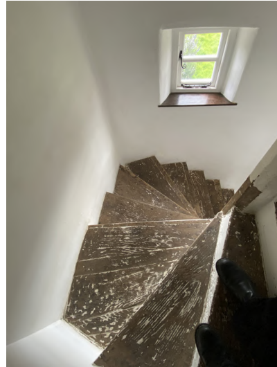
Newel post on the right of the image usually found in more prosperous houses and often as here rises through more than one storey to serve the attic as well.
