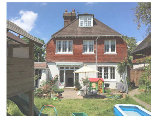
Reference Point Photo showing the clear tonal and material horizontal split to the existing rear elevation
