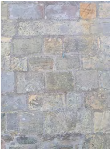
Figure 6 Evidence of blocked window (supplied by client)
