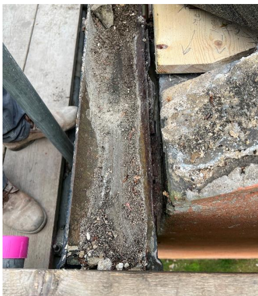
Fig 1. Existing gutter corrosion.
