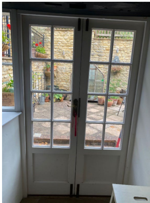
Internal view looking out over the patio and the step down to the French doors, which creates a flooding issue during heavy rainfall
