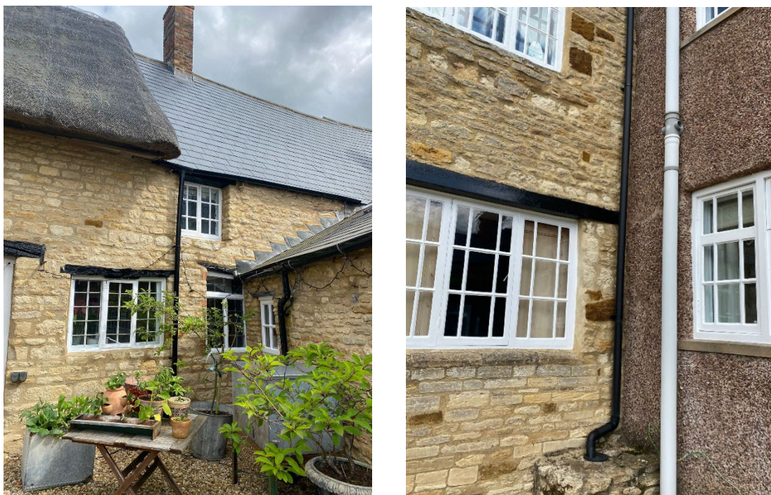
Example of current UPVC rainwater goods, to be replaced with either cast iron or heritage aluminium RWG
