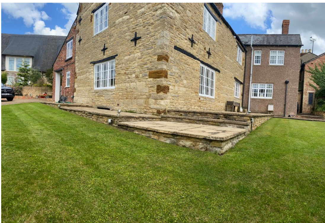
Photograph showing the elevated concrete-paved patio to the south and west elevation to be removed and reinstated to grass, with a 900mm wide ground-level path around the perimeter of the property.
