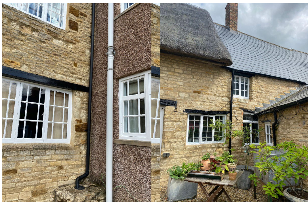
Example of current UPVC rainwater goods, to be replaced with either cast iron or heritage aluminium RWG
