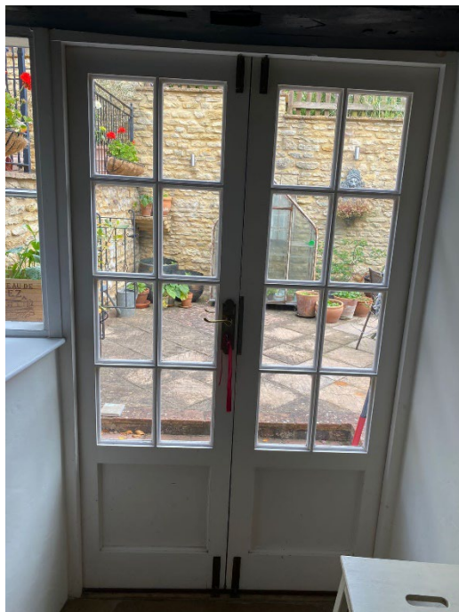
Internal view looking out over the patio and the step down to the French doors, which creates a flooding issue during heavy rainfall
