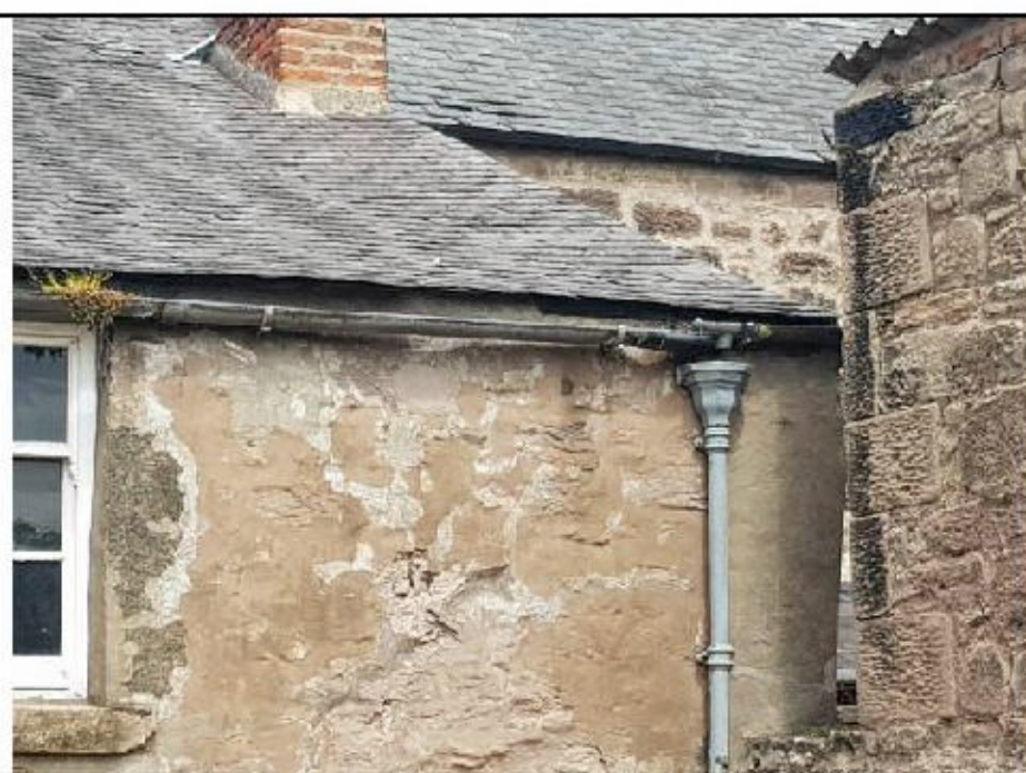
Photograph 6. Section of missing mortar at eaves height behind drainage stack.
