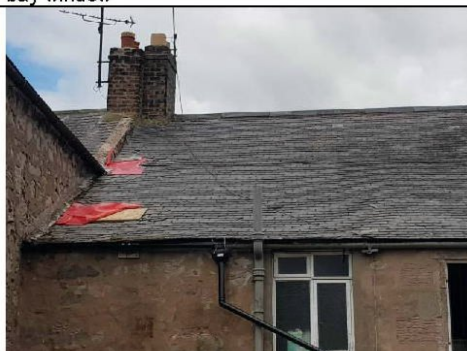
Photograph 4. Roof tile damage at rear
