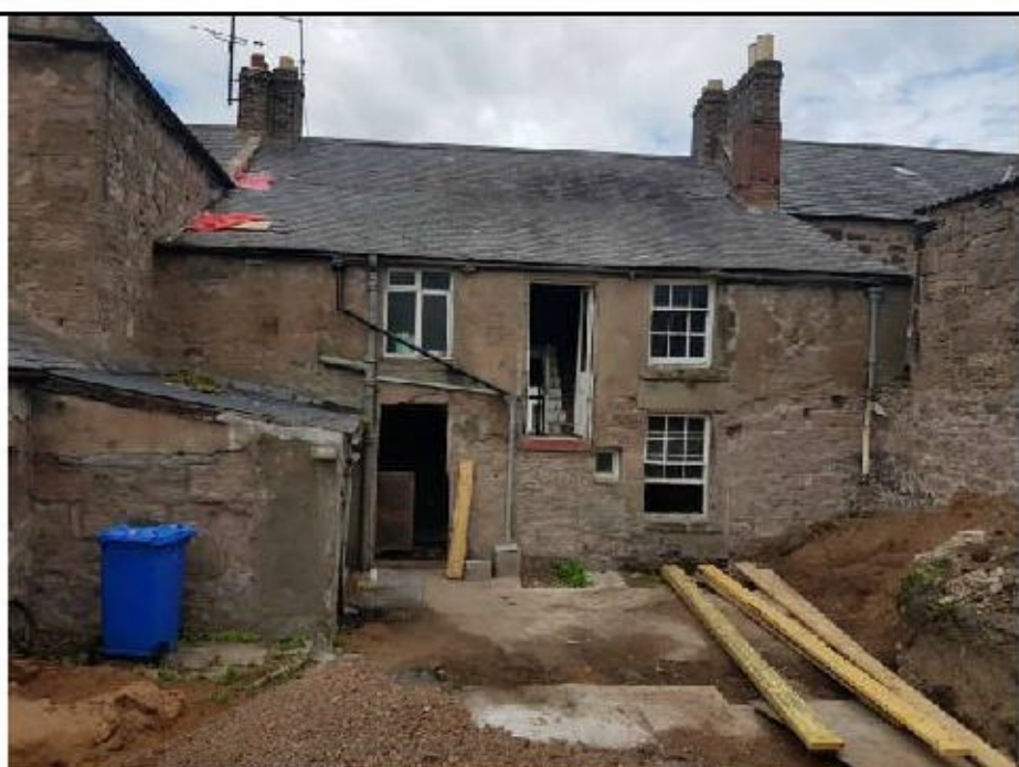
Photograph 3. Rear of property. Staircase below central window and built structure to right of image have been removed. Shallow mortar gaps can be seen
