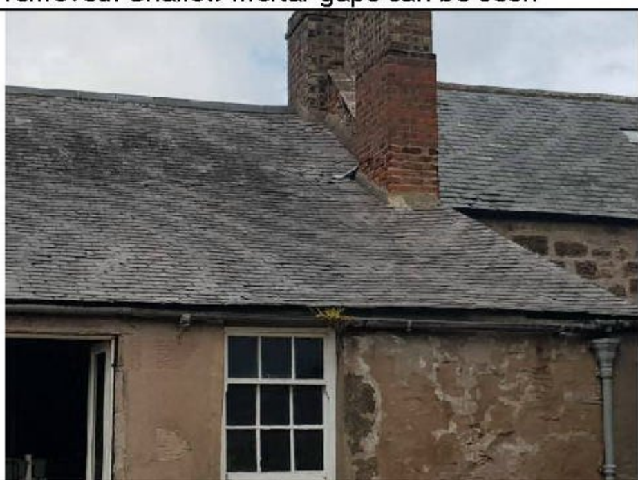
Photograph 5. Examples of slipped and lifted tiles as well as lifted lead flashing at rear
