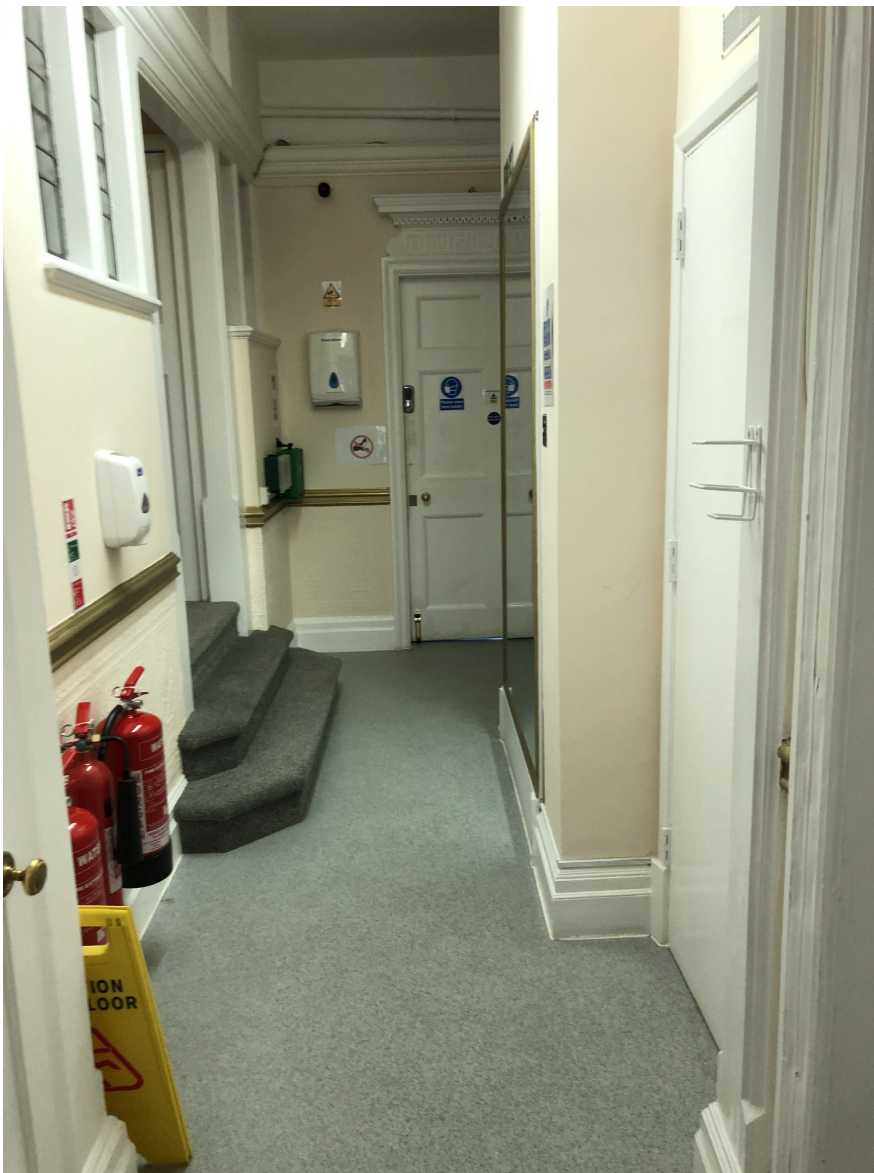
Typical intrusion of lift into circulation space, inadequate for modern clinical useage.
