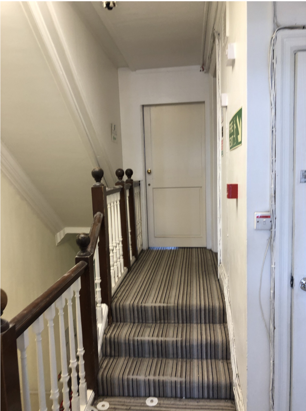
Limited circulation space for clinical use due to lift
