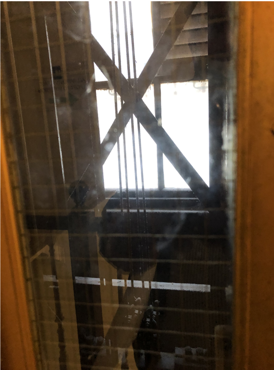
View of redundant lift mechanism through glazed lift door. Original window to lightwell beyond
