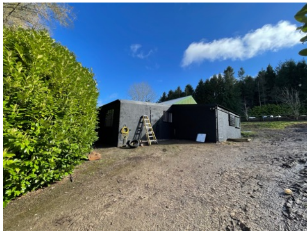
Photograph 8: View of the southwest corner of the building with Section C attached to the west elevation.
