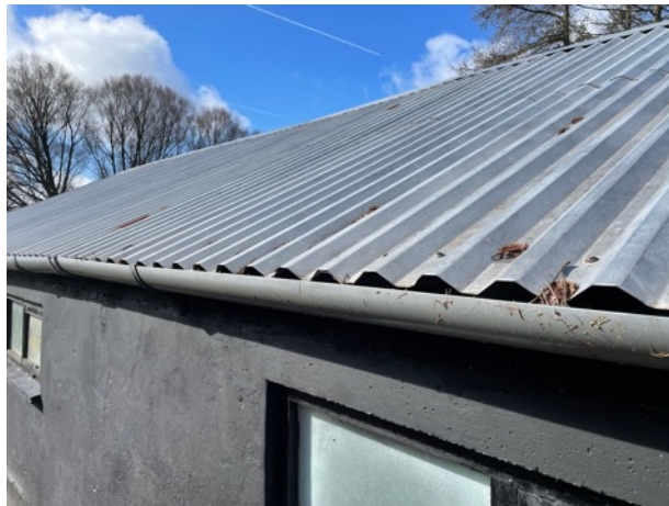
Photograph 15: Gaps along the bottom of Section B corrugated roof.
