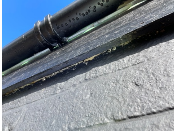
Photograph 13: Gap behind the timber fascia board of Section A.
