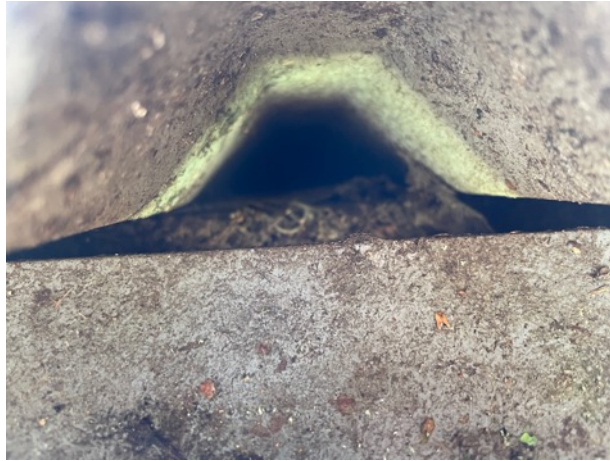
Photograph 19: Gaps along the corrugated roof of Section D.
