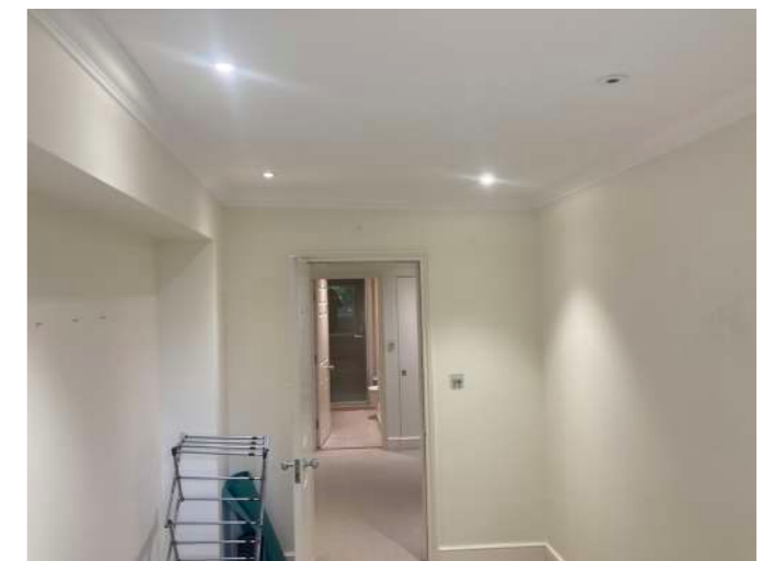
Figure 59: Existing lighting to ceiling in Bedroom 3.
