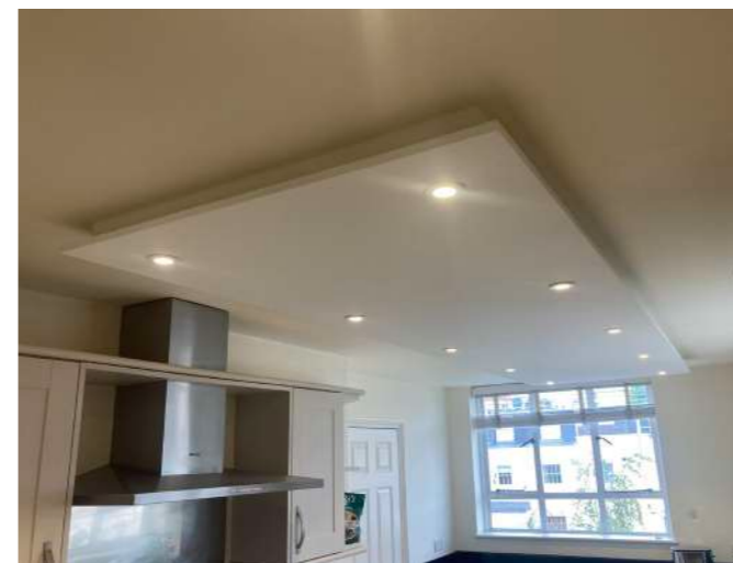
Figure 58: Existing lighting to ceiling in Kitchen. The unsightly dropped ceiling will also be removed.
