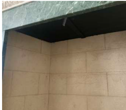
Figure 52: Existing Dining Room top of chamber blocked up.
