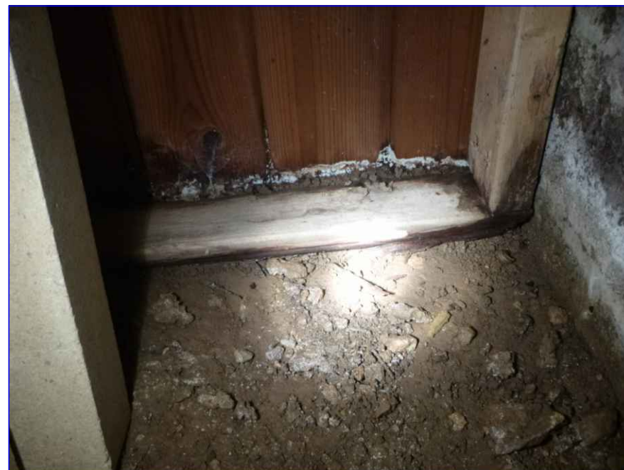
Photograph 4: Showing the timbers at the front of the bat roost which are beginning to rot.
