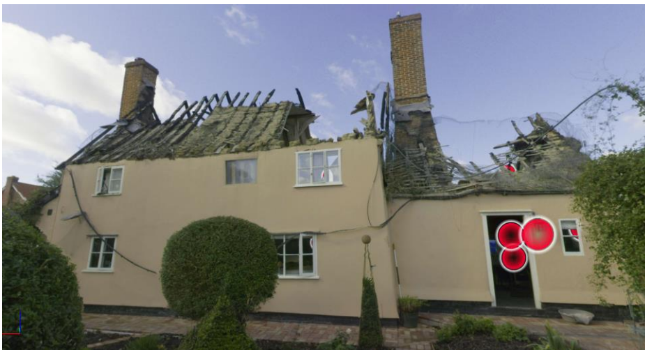
Front and rear photos showing fire damage
