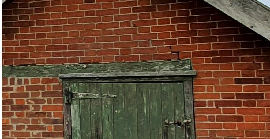
Figure 30 – Cracking above weathered timber lintel
