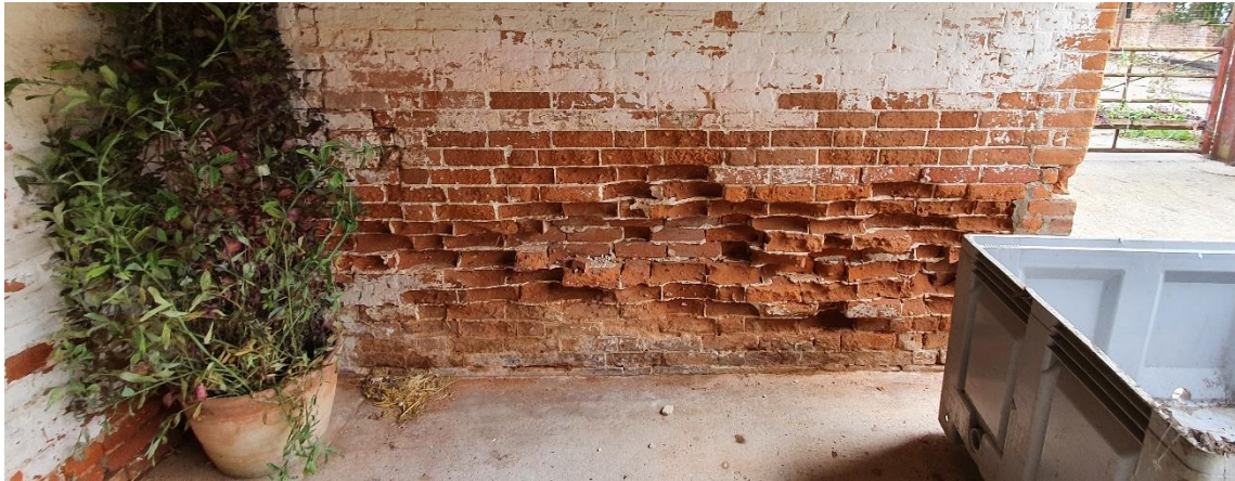
Figure 35 – Significant damage to masonry wall
