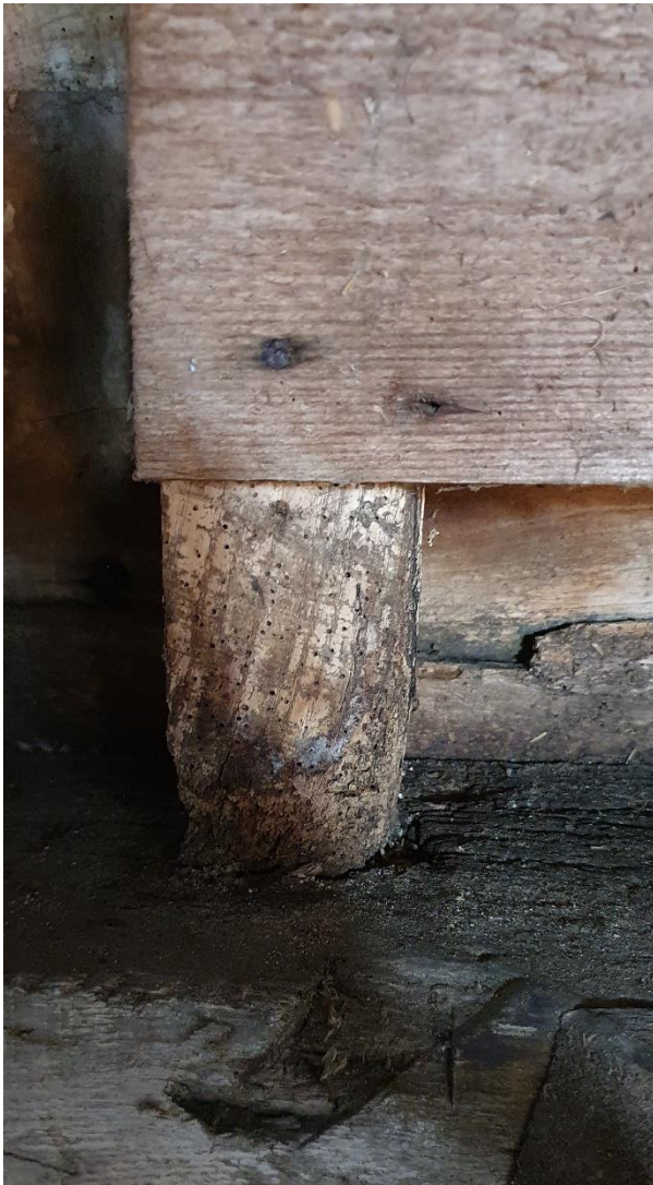
Figure 38 – Typical timber defects to barn 3
