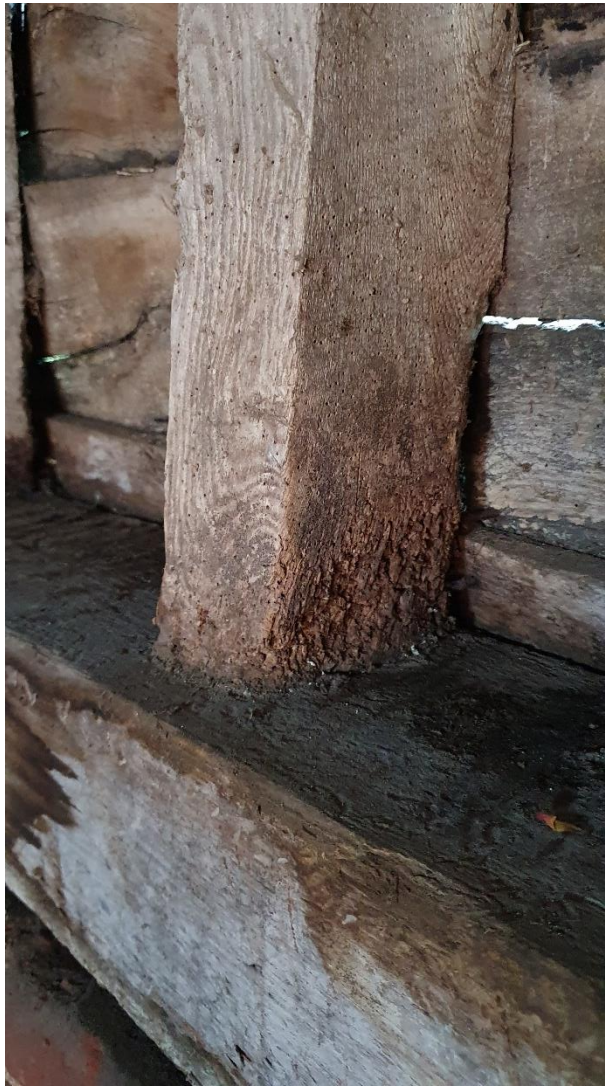
Figure 39 – Further typical defects to barn 3
