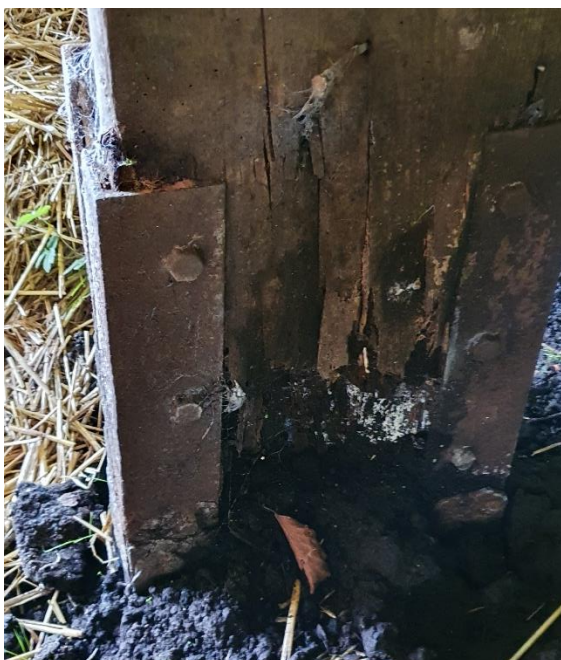
Figure 9 – Significant rotting of timber columns
