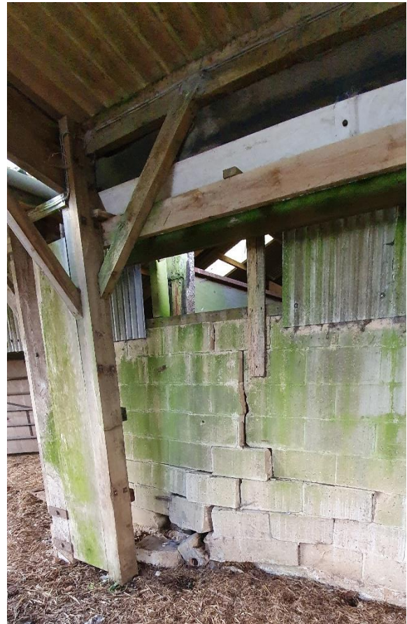
Figure 8 – Damage to external wall to rear of barn
