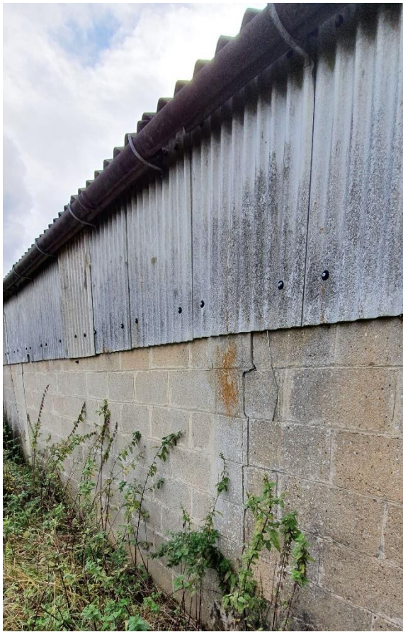
Figure 7 – Vertical cracks at portal frame locations
