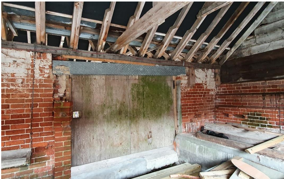
Figure 36 – Removal of masonry directly below lintel bearing. Note drop in lintel at support.
