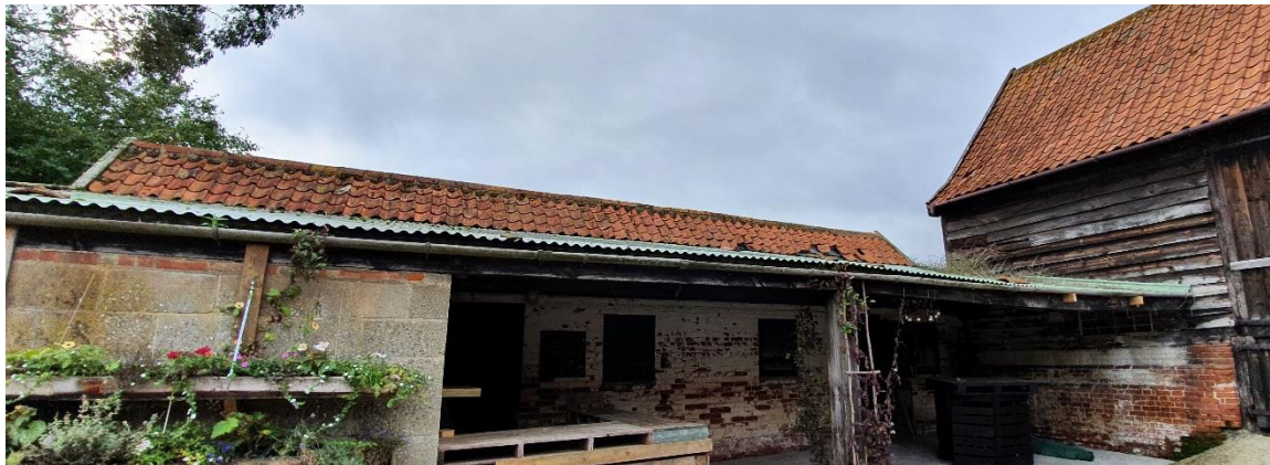
Figure 34 – Outbuilding with lean-to roof. Note lack of flashing between both roofs
