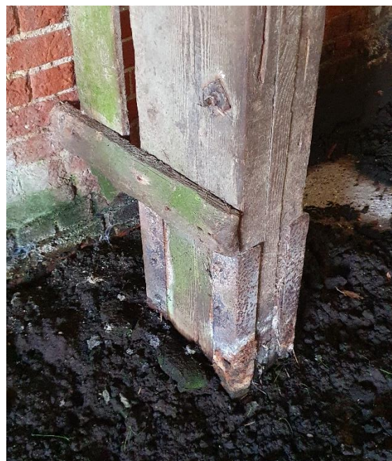
Figure 10 – Corrosion of both timber and steel
