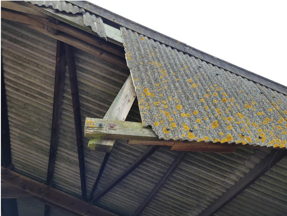
Photograph 3 – Asbestos seen on the front of barn 7.
