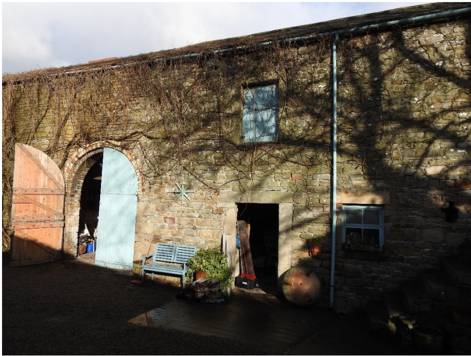
Ling Villa barn south elevation as existing showing later addition brick arch and vertical joint at change in stonework
