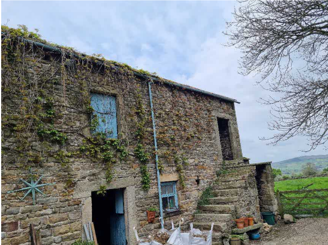
Image 19 – southern elevation of B1 showing stairs which lead to entrance to loft void
