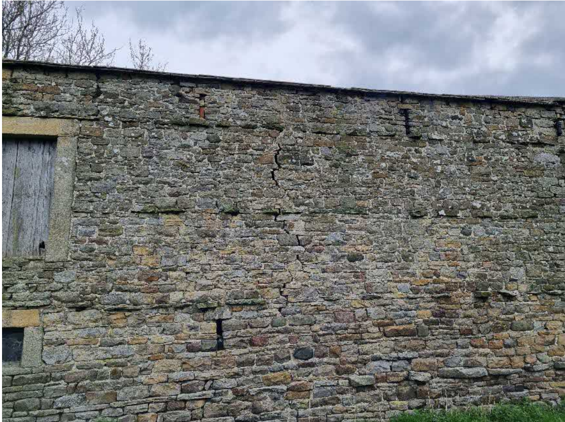
Image 11 – northern elevation of B1 showing PRFs in brickwork
