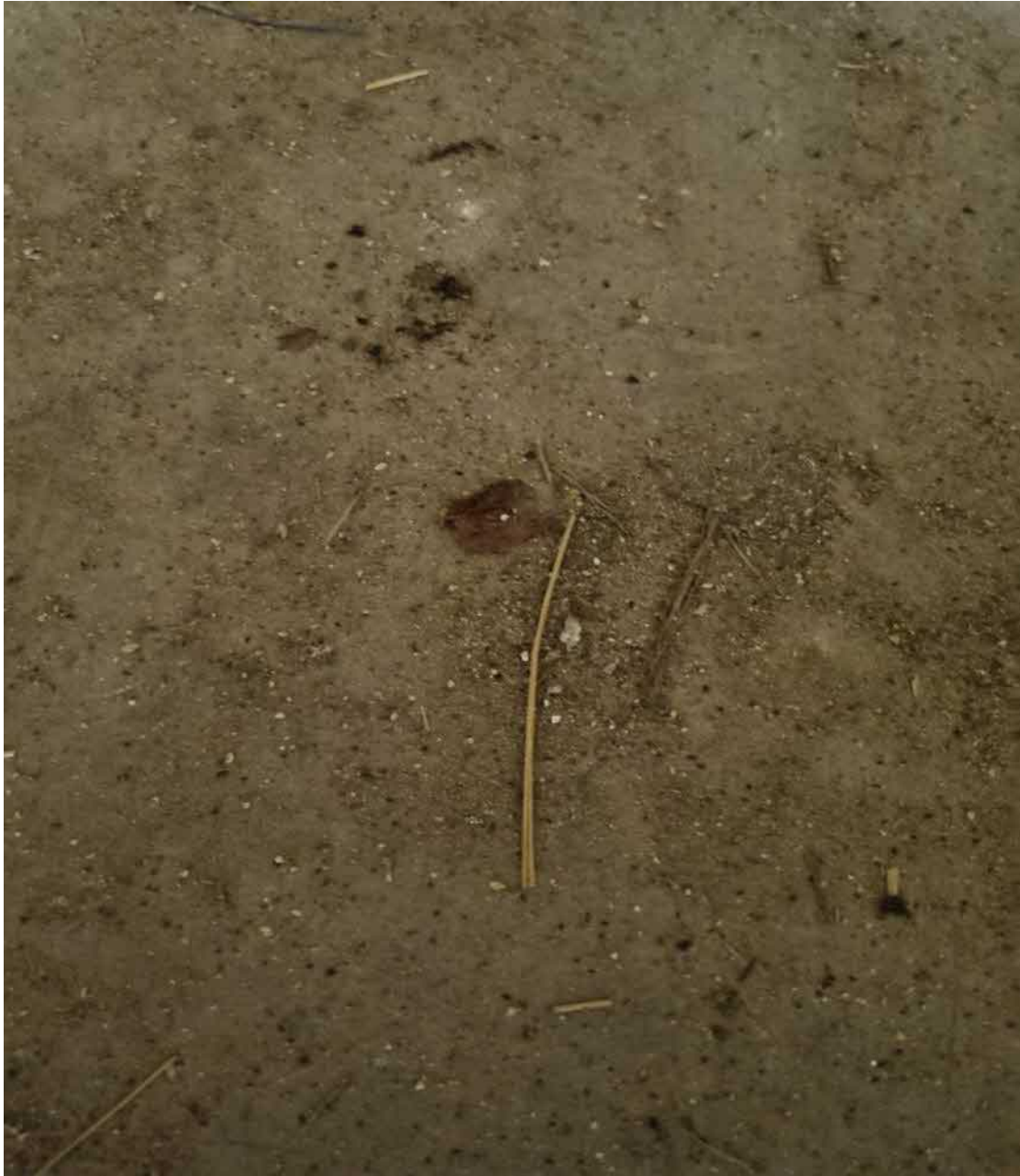
Image 3 – bat faeces on floor of eastern end of loft void
