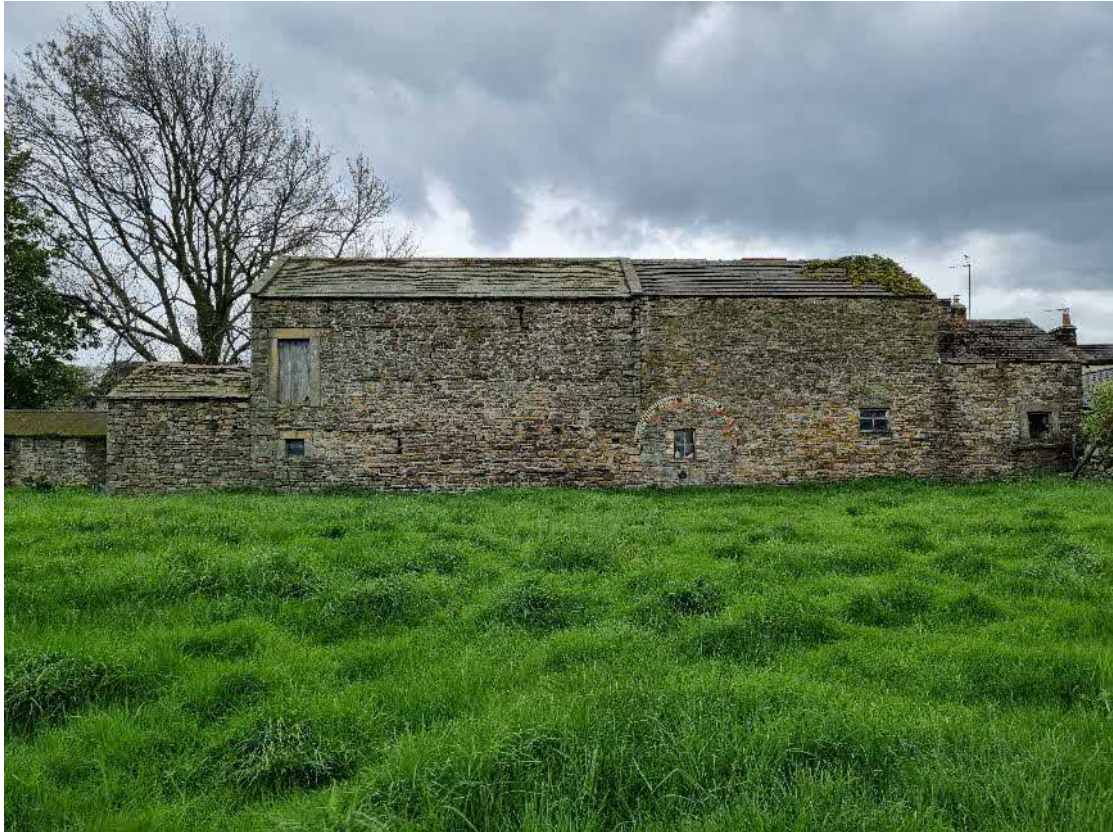
Image 25 – northern elevations of B1 and B2 showing multiple PRFs in brickwork and roofing
