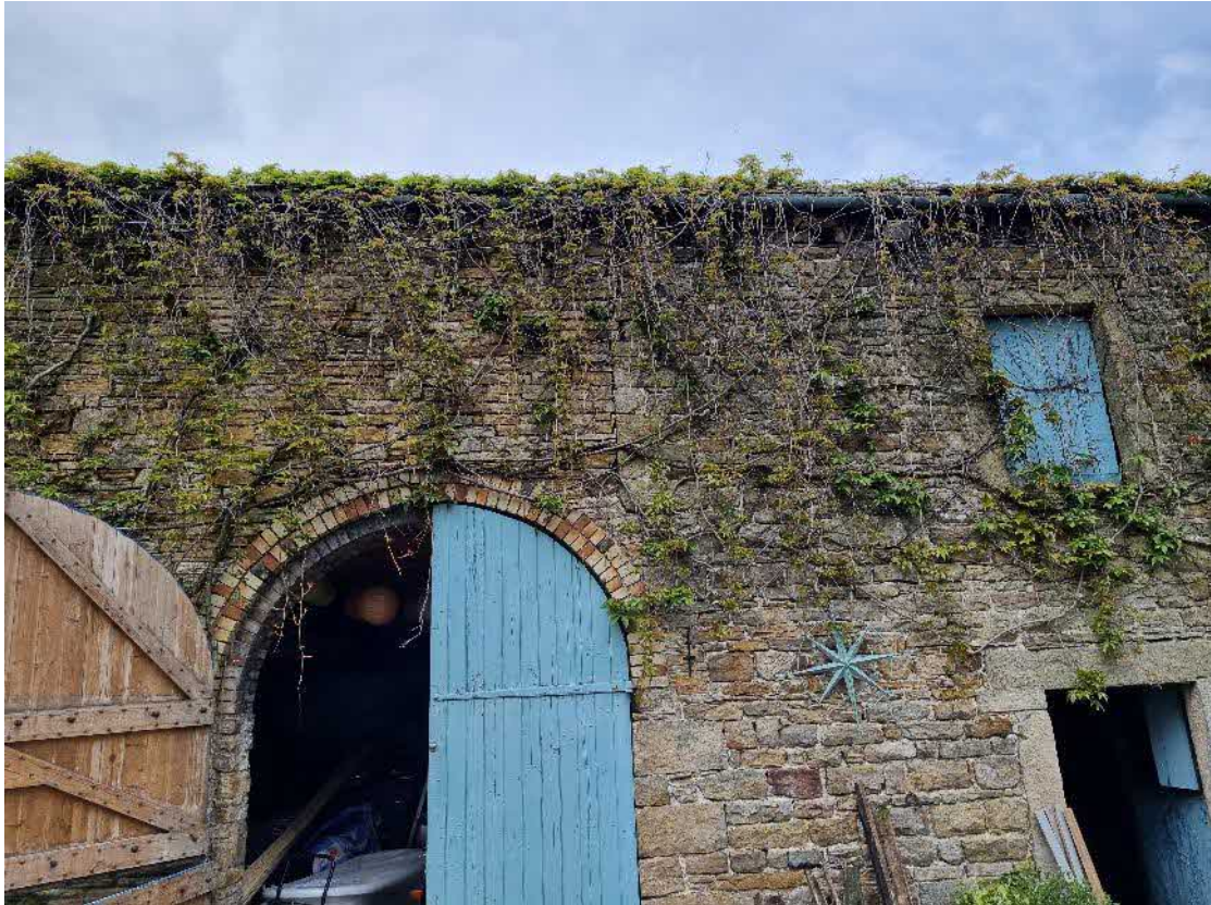
Image 18 – southern elevation of B1 showing PRFs visible in brickwork. House sparrows also utilising gaps in brickwork for nesting
