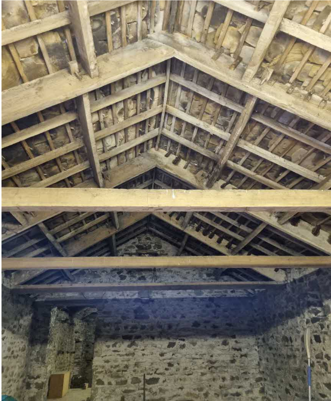
Image 2 – internal loft void space at eastern end of B1 showing wooden beams
