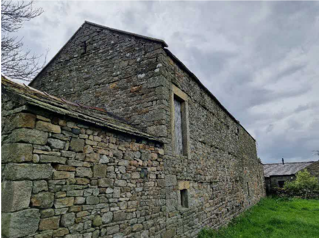
Image 10 – external view of northern and eastern elevations of B1, showing PRFs externally in brickwork and under roofing
