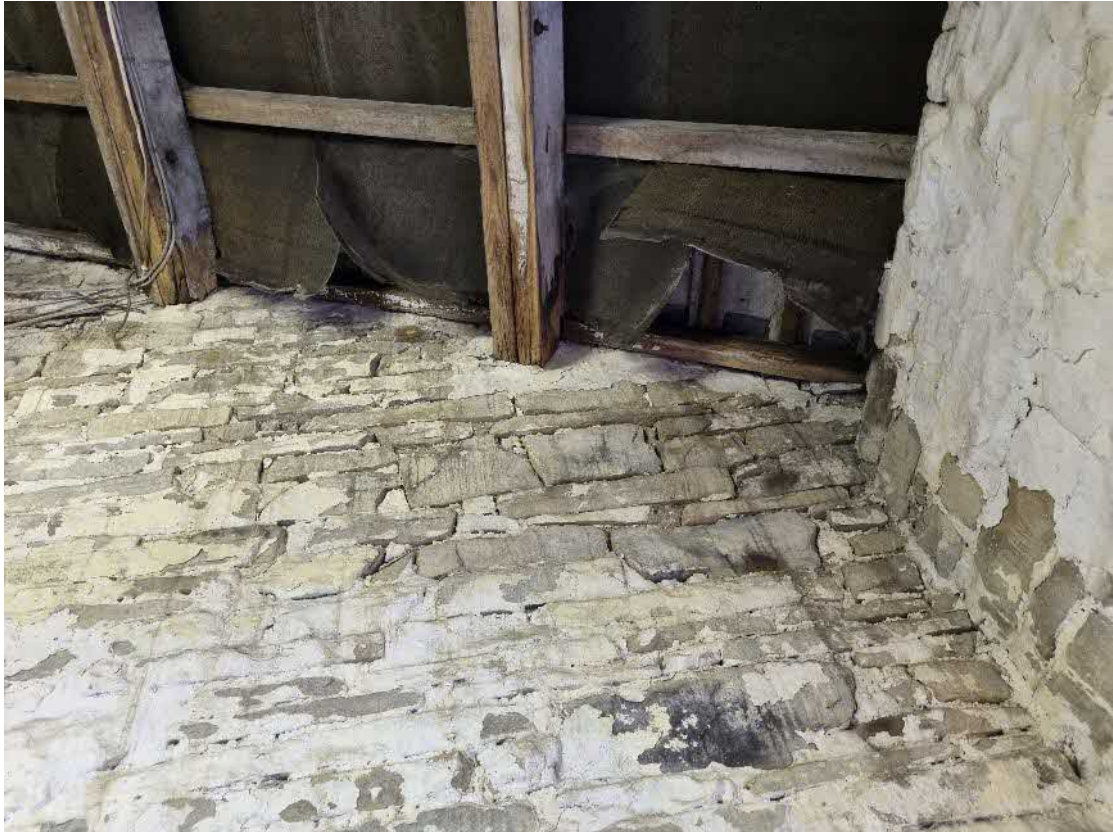
Image 20 – gap in roof felting exposing PRFs.
