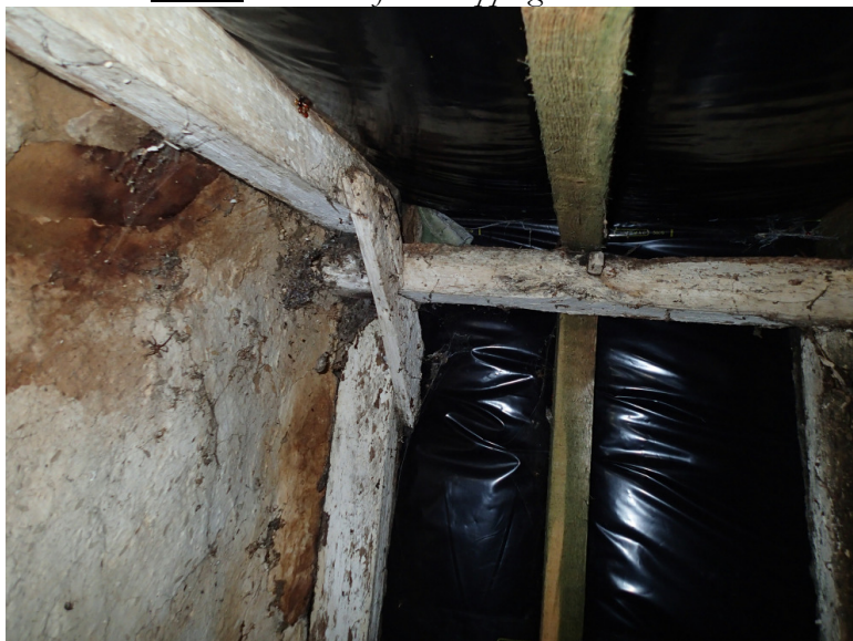
Photo 3 Location of bat droppings in attic room
