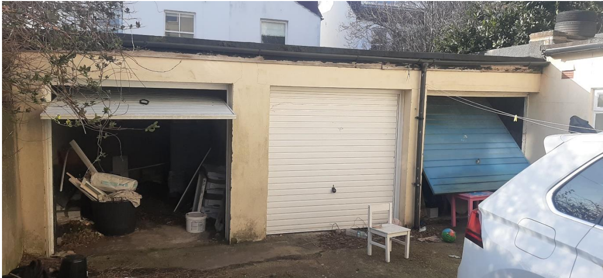
Photograph 01: Dilapidated unused garages.
