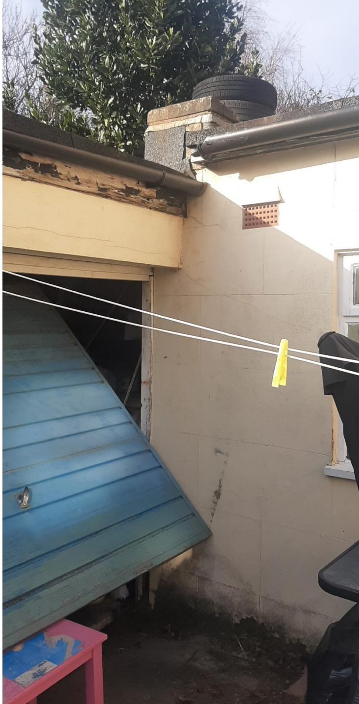
Photograph 03: Dilapidated unused garage with broken garage door Propped open giving onto kitchen window of number 14 Ground Floor Flat
