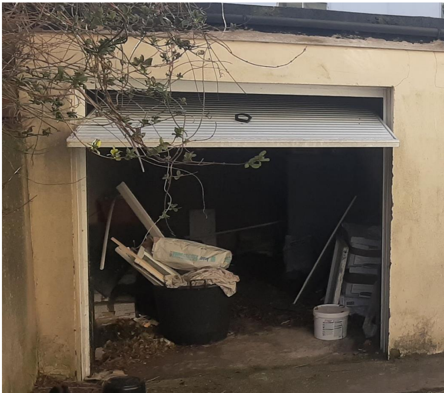
Photograph 02: Dilapidated unused garage filled with storage items
