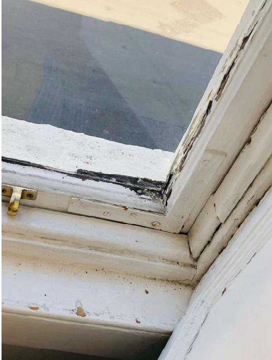
Metal brace holding window together
