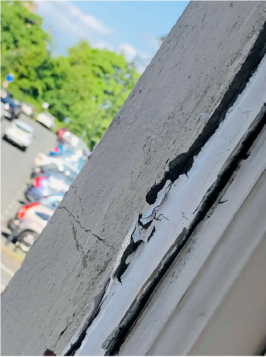
More rotten timbers
