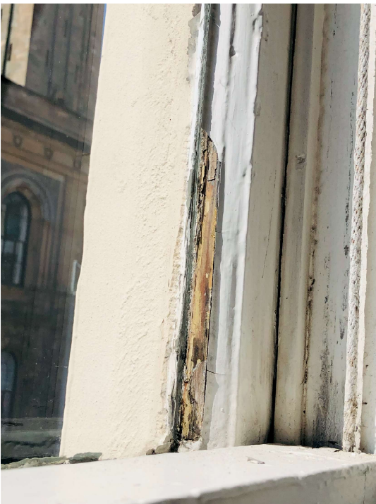
More rotten timbers
