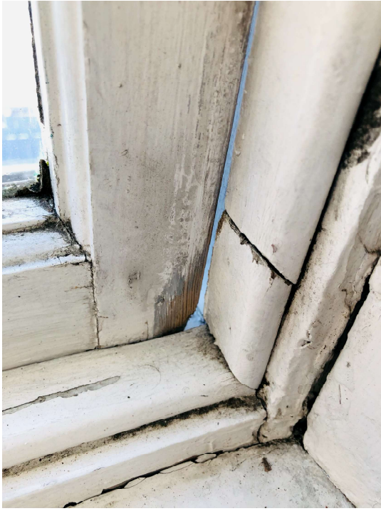
Hugh gap left from sash being too small. This was a replacement as the original had rotted so bad
