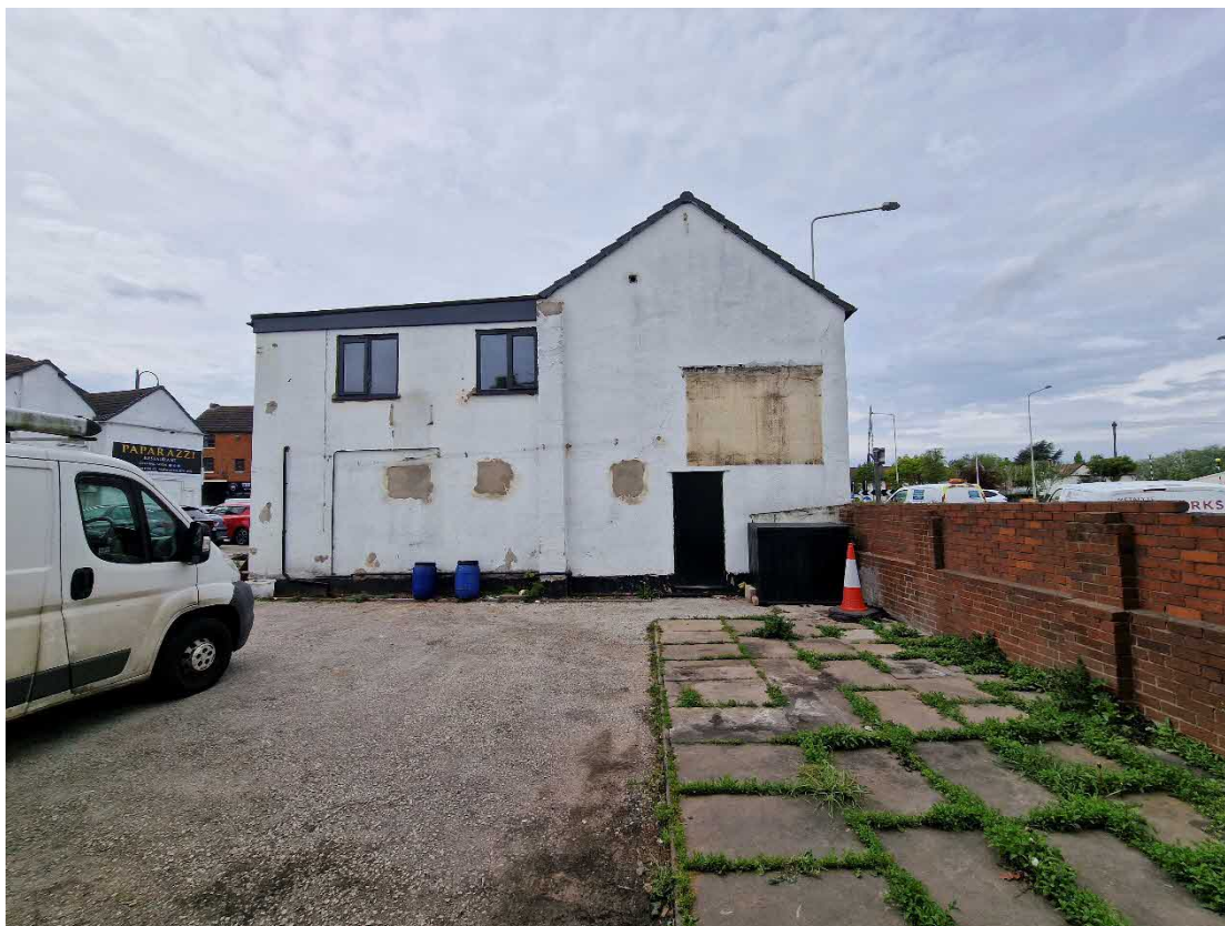
Plate 15: East gable elevation and flat-roofed west extension to the rear car park
