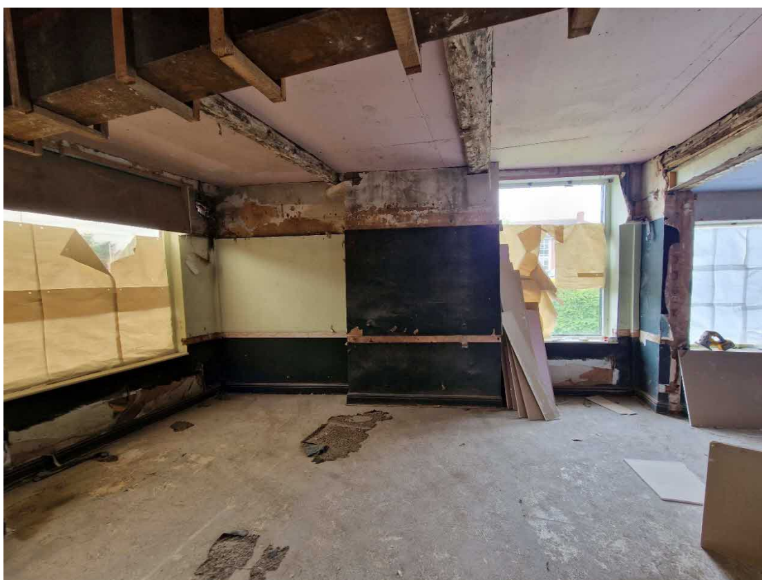
Plate 20: Northwest corner of the restaurant with windows to Coleshill Street and Atherstone Street
