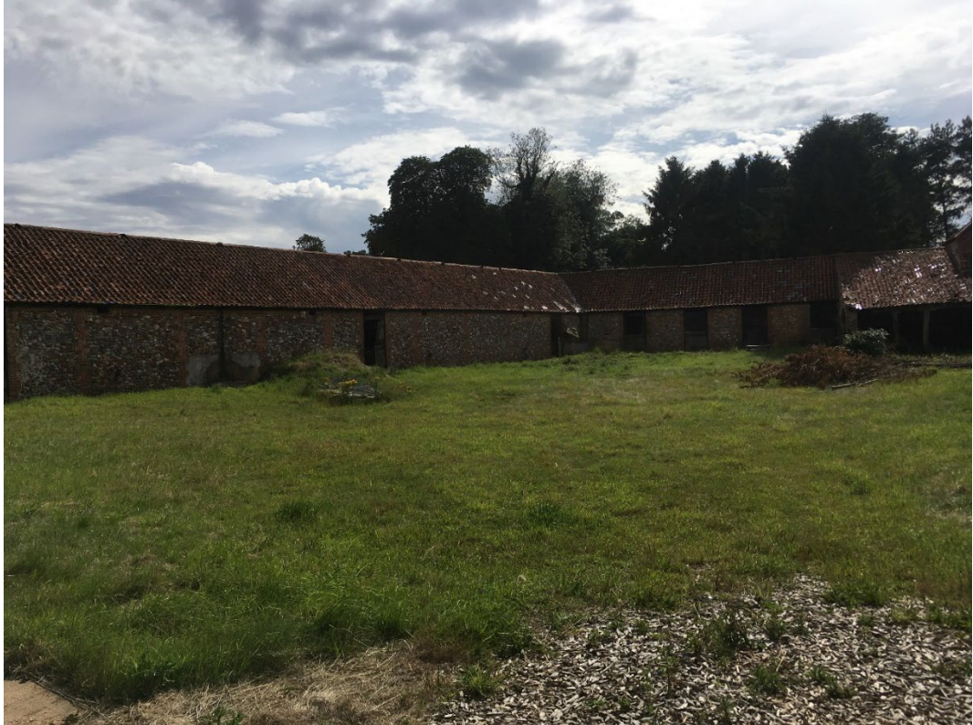
Image 4 (above): Northern elevation of southern wing and eastern elevation of Western Wing
