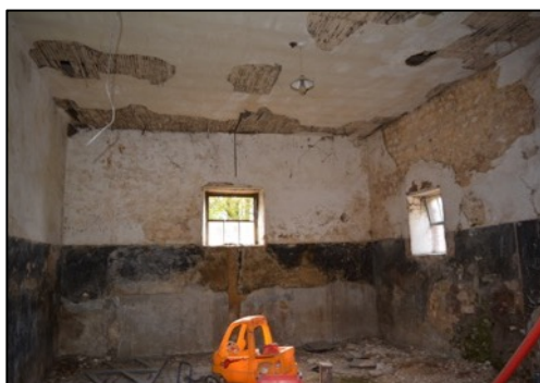
Figure 28 – Internal view of Main Barn 4 Complex (Section I) showing the lath and plaster ceiling including gaps
