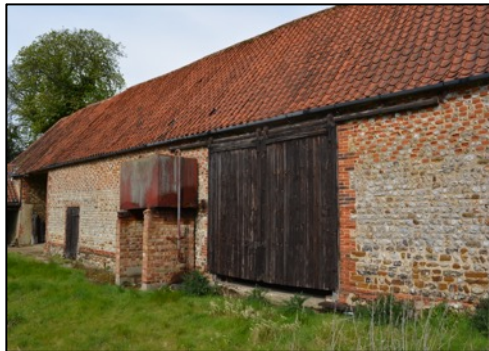
Figure 15 – Western elevation of Main Barn 4 Complex showing a wooden access door where gaps were present
