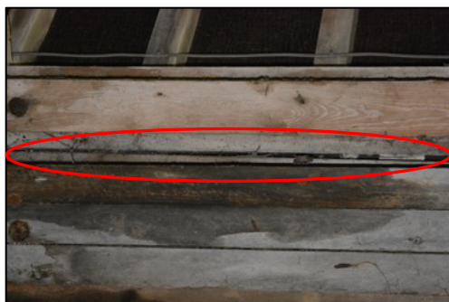
Figure 34 – Feature between the lintel and door frame that a barbastelle was found on the eastern elevation of Barn C
