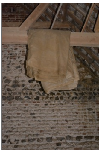
Figure 40 – Hessian sack over the rafter where a brown long-eared was recorded roosting during the 2020 bat activity survey (20 th August 2020)
