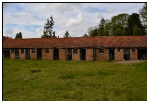
Figure 19 – Southern view of Main Barn 4 Complex (section J), showing the damaged doors and windows
