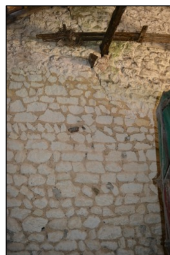
Figure 46 – Cavities in the chalk wall of the trailer store
