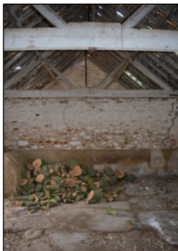
Figure 26 – Internal view of Barn 4 Complex (section F), showing its poor state of repair
