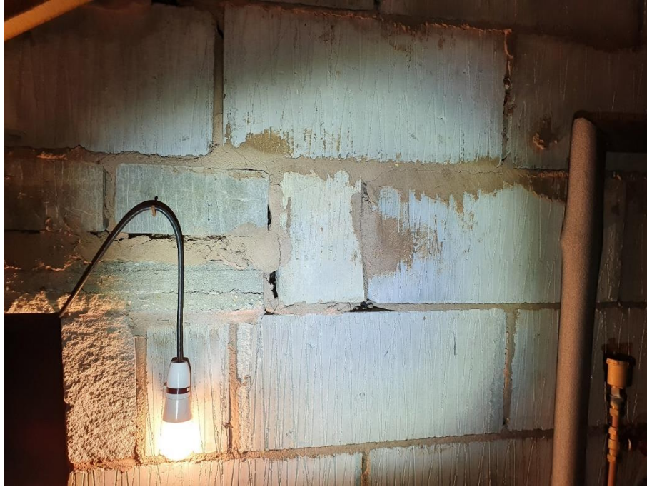
Figure 4.9. Holes in wall
