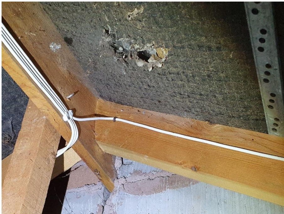
Figure 4.8. Hole in lining
