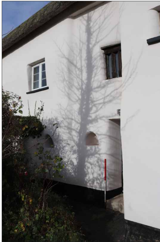
Plate 4: Bee boles in south elevation of the farmhouse, looking northwest, also showing an early window over the cross passage (1m scale)
