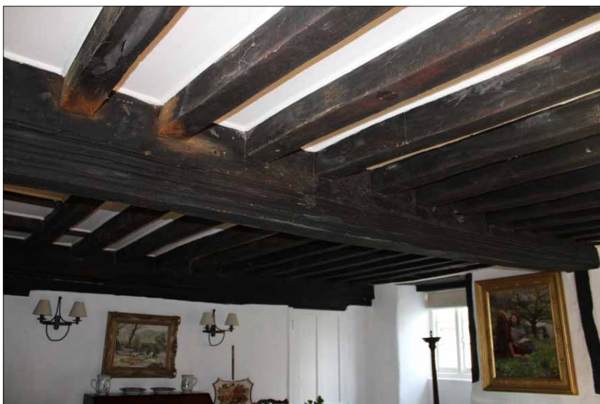
Plate 9: Central bridging beam in the hall, looking northwest with the replaced partition to the cross passage in the background
