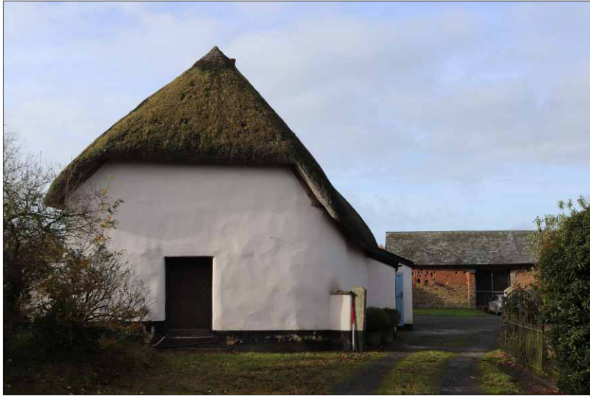
Plate 7: East elevation of the farmhouse, with the threshing barn in the background, looking west (1m scale)
