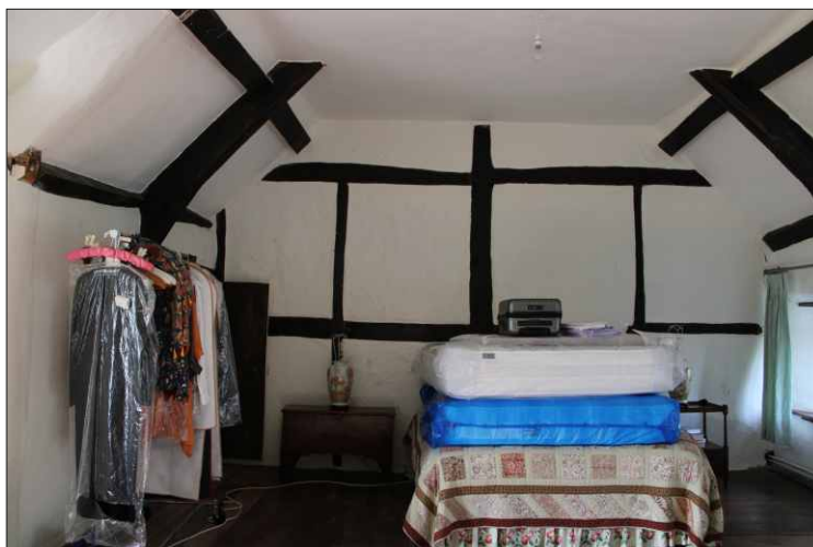
Plate 24: Timber-framed partition between bedrooms 3 and 4, looking west from within bedroom 3, looking west
