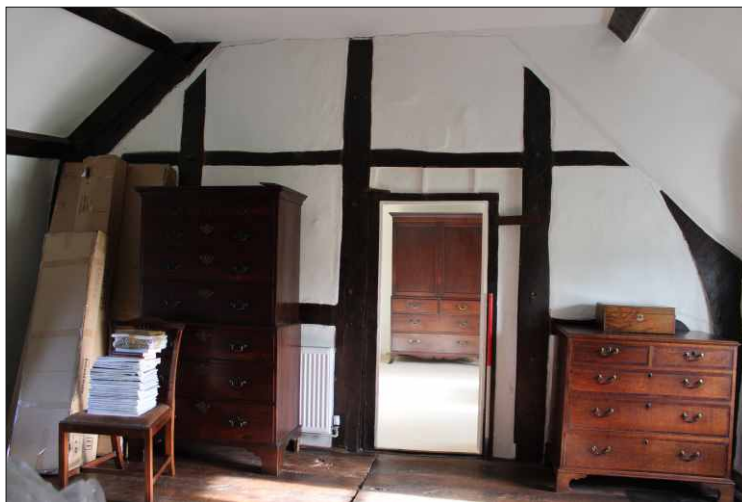
Plate 23: Timber-framed partition between bedrooms 2 and 3, looking east from within bedroom 3 (1m scale)
