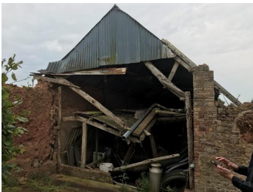
Missing sections of structure and ad-hoc flimsy repairs no longer allow safe use
