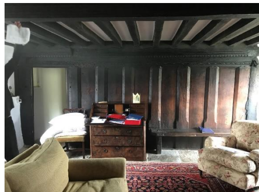
Careful removal of inappropriate finishes to historic timbers and like for like conservation repairs to internal features.
