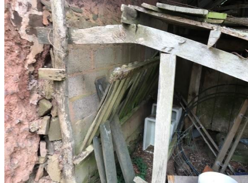
Feeding stall to Linhay with concrete block repairs to cob walling to be retained and cob junction consolidated.
