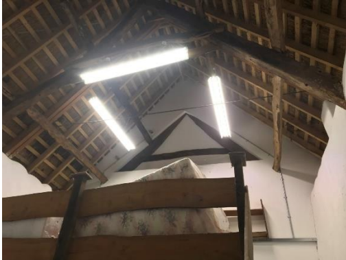
Roof structure over Shippon Mezzanine to have soffit installed below modern rafters keeping the historic timber exposed.
