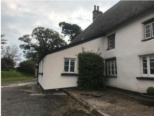
Kitchen block with modern casements to be replaced and concrete platform to be removed and ground made good.
