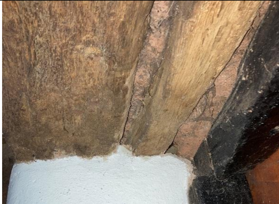
Photo 14: Internal gaps around door lintel.
