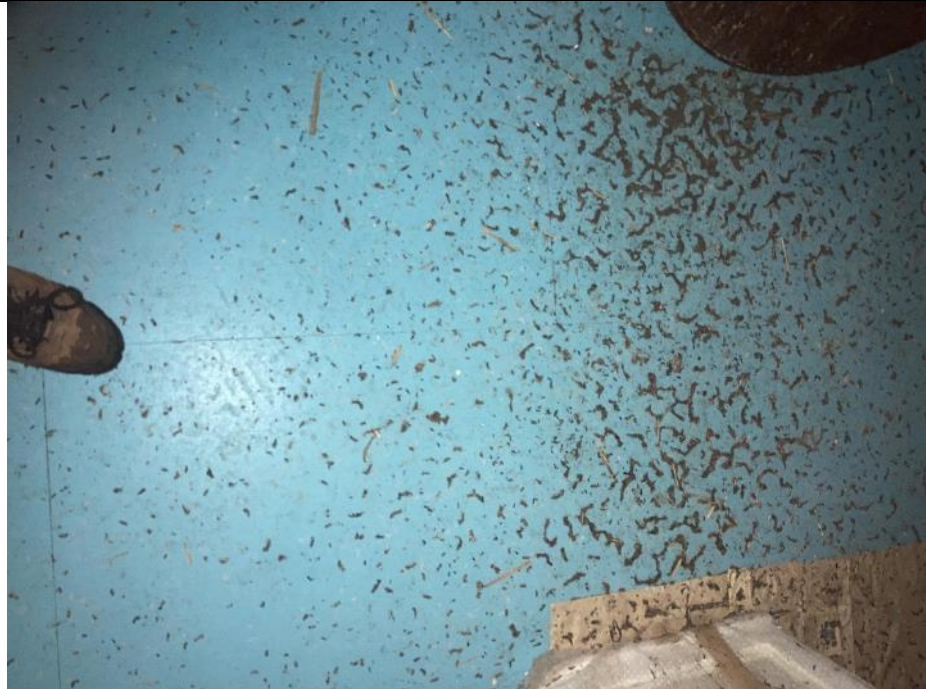
Photo 16: Example concentrated bat droppings beneath ridge.
