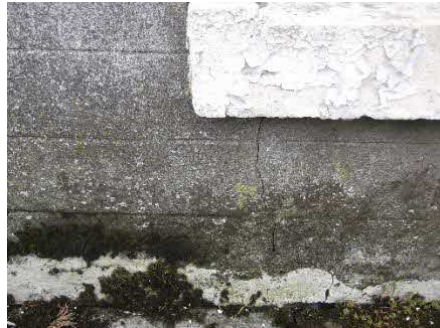
Cracking Under Cill
