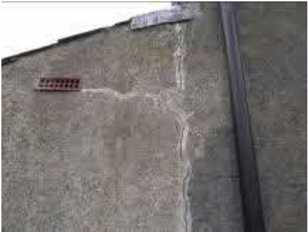
Gable Wall Cracking
