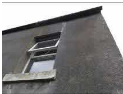
Major Crack at Eaves
