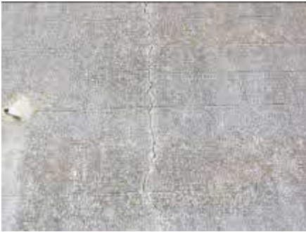
Major Crack Full Height of Gable
