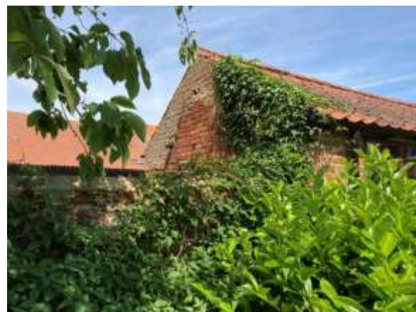
Gable return, note raised masonry
