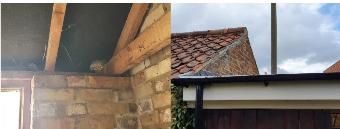
Fig 9. Torn internal lining (left) Fig 10. North gable end, partially obscured by lean-to polycarbonate roof
