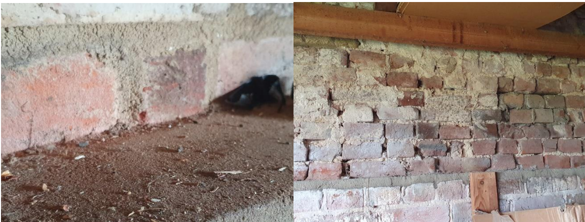
Fig 7. Droppings observed on window sill (left) Fig 8. South gable wall internal (right)
