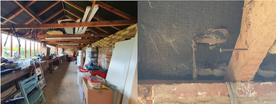
Fig 5. Internal view of barn (left) Fig 6. tear in internal lining (right)
