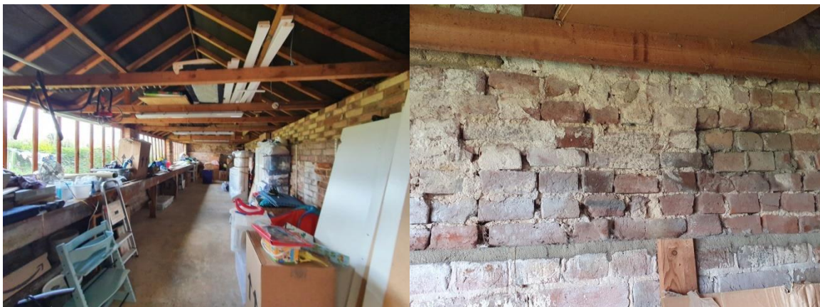
Fig 6. Internal view of building (left) fig 7 Some shallow brick cracks in internal walls (right)
